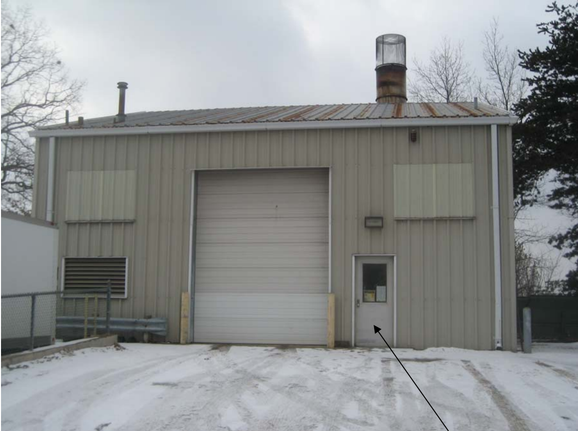
#2 Assumed Fire Door and Frame
