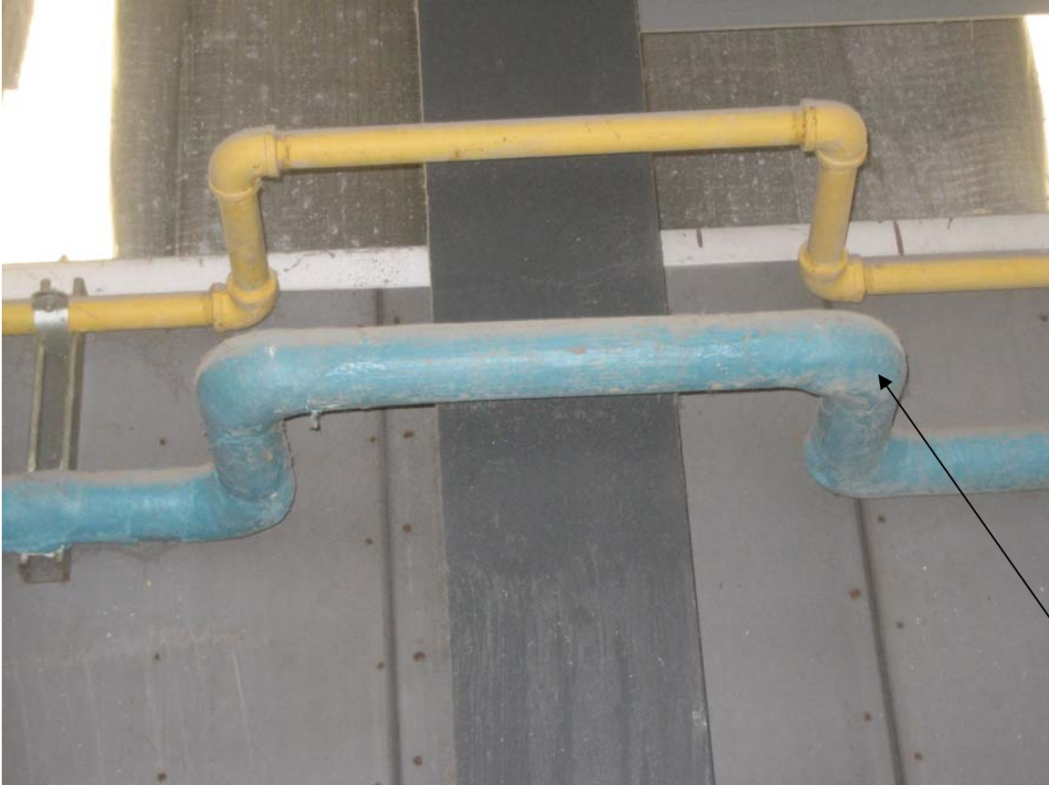
HA #1 – Non asbestos containing mud fittings on fiberglass
