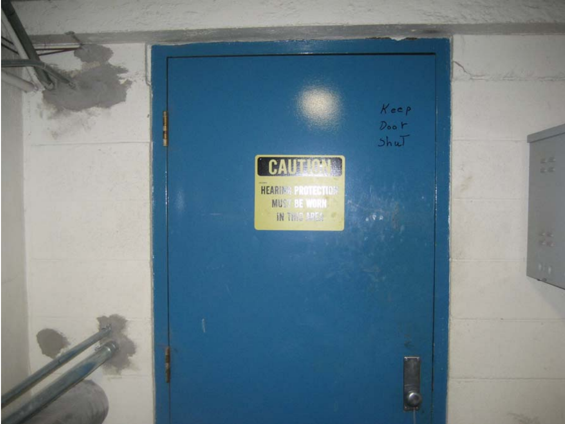
HA #5 – Assumed asbestos containing fire door and frame
