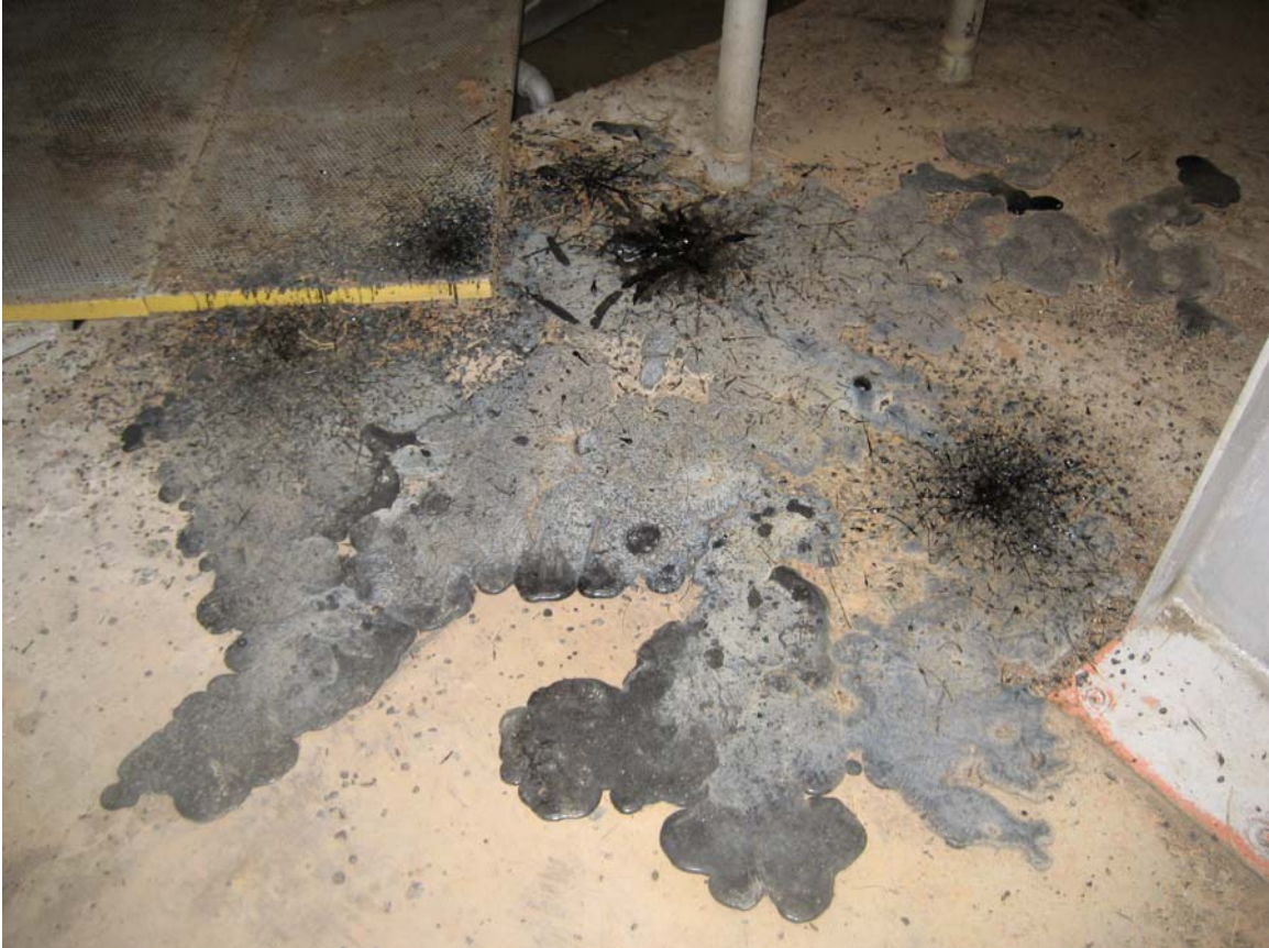
HA #7 – Non asbestos containing melted tar material
