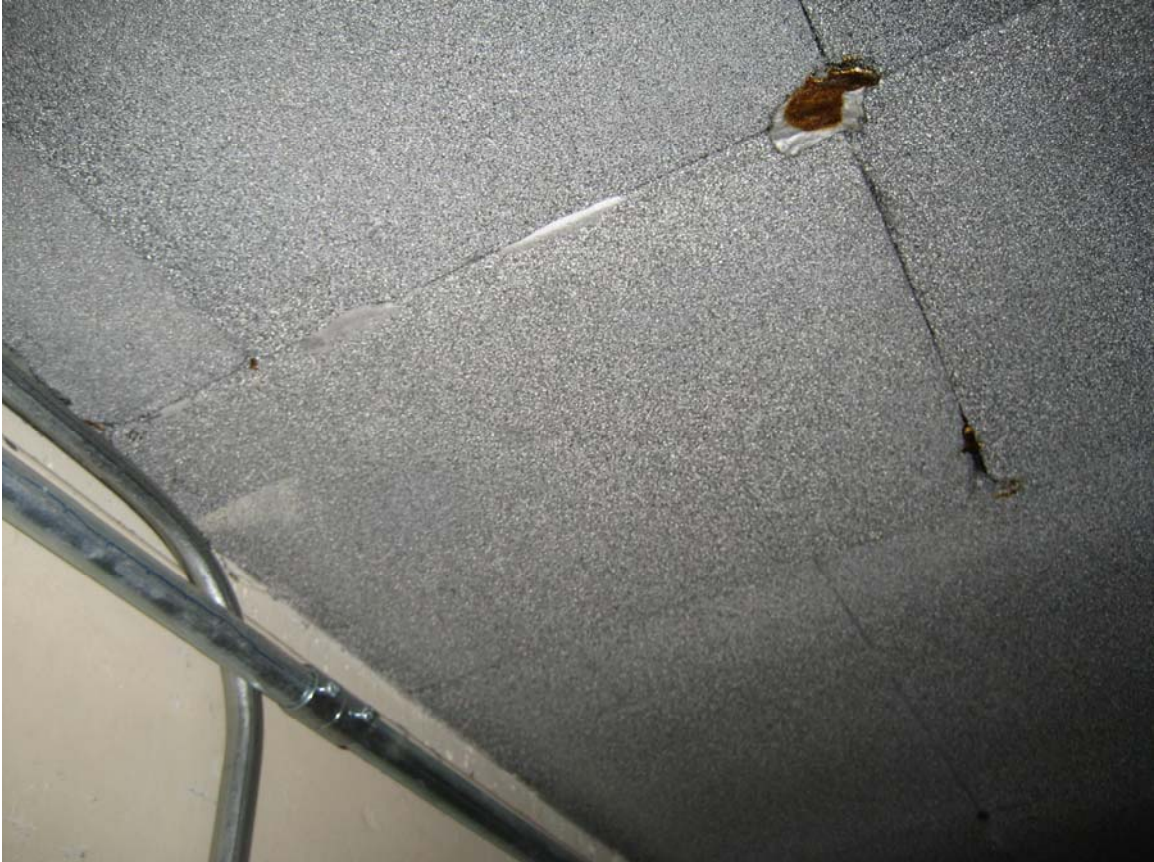
HA #1 – Non asbestos containing Gray Styrofoam insulation and associated brown gluepods
