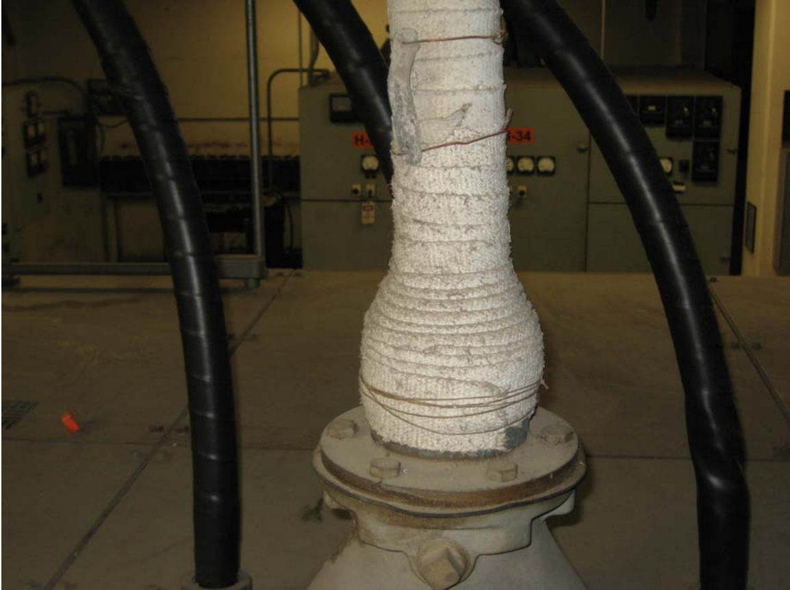
HA #3 – Assumed asbestos containing white electrical line wrap
