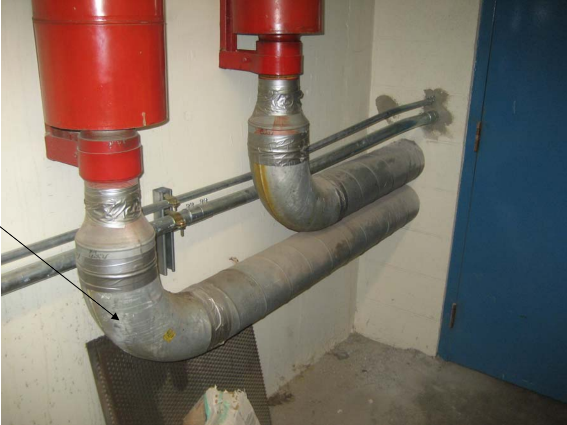
HA #10 – Assumed asbestos containing 0”-12” metal jacketed steam line
