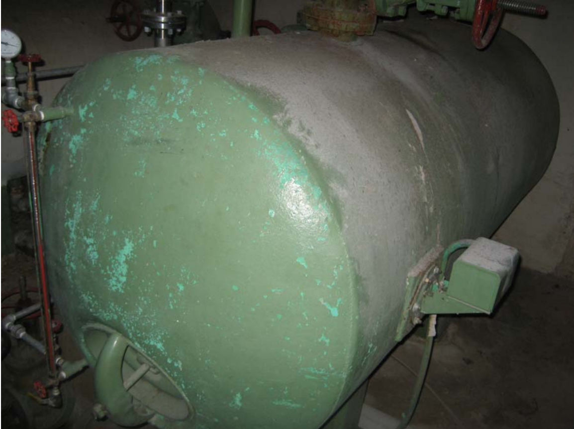
HA #8 – Assumed asbestos containing tank insulation
