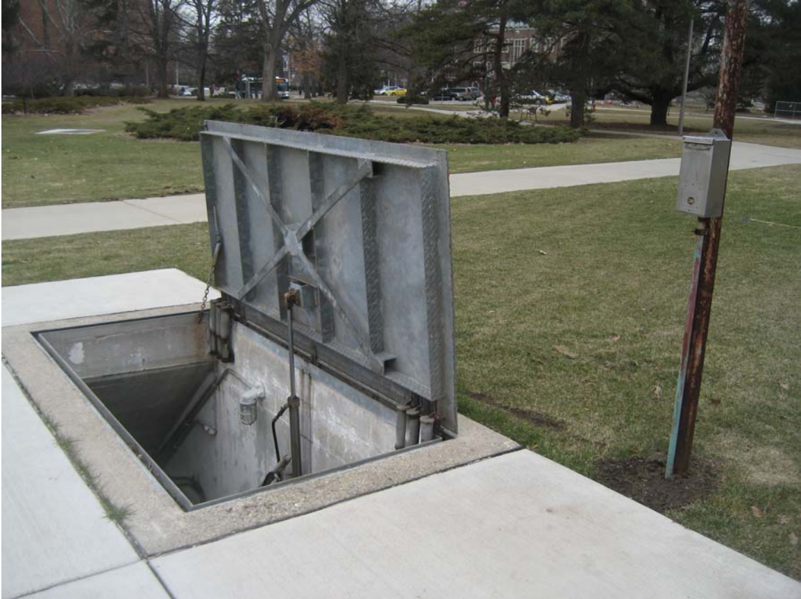
North Campus Substation (#516)
