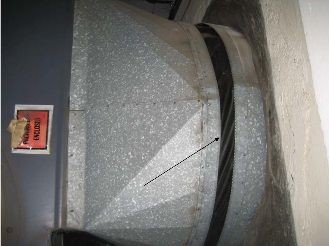
HA #2 – Assumed asbestos containing vibration collar
