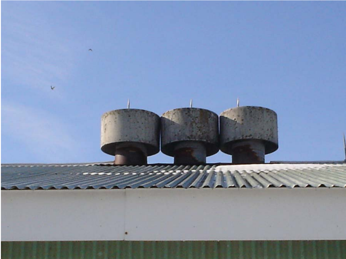
HA # 18 – Assumed asbestos containing transite roof vent covers
