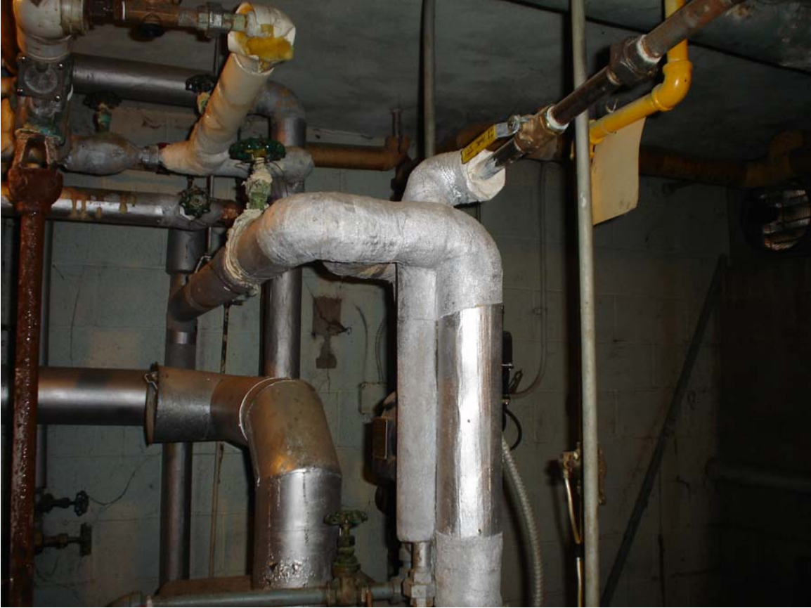
HA #8 – Asbestos containing steam/condensate supply and return pipe joint and hanger insulation
