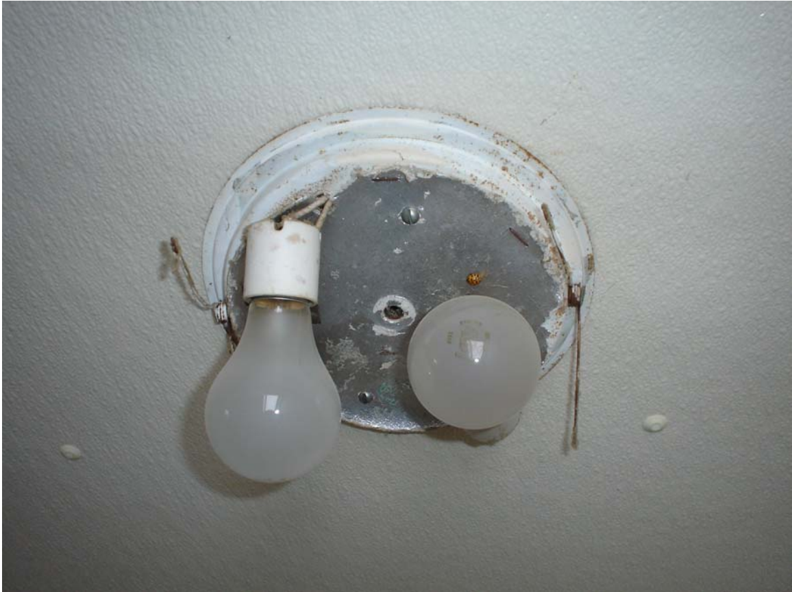
HA #6 – Asbestos containing light heat shield insulation
