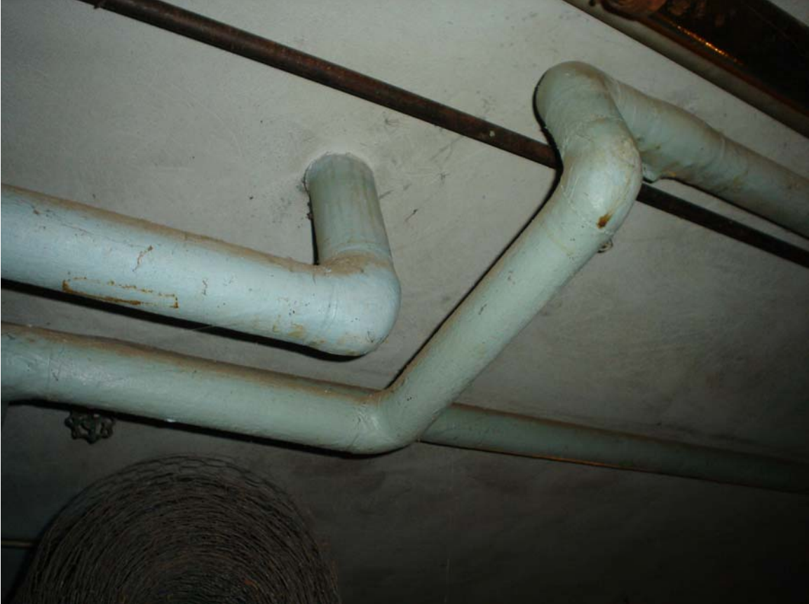
HA #9 – Asbestos containing domestic water supply pipe joint and hanger insulation
