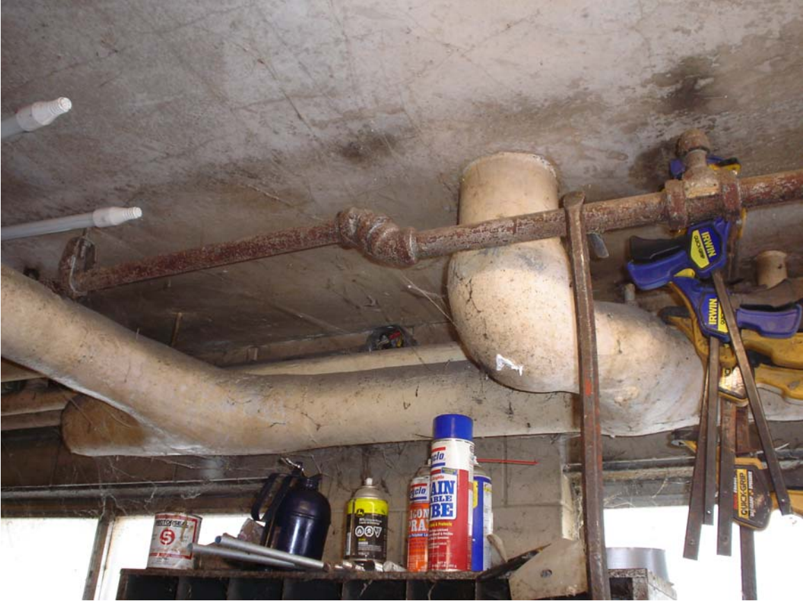
HA #11 – Asbestos containing drain line pipe joint and hanger insulation
