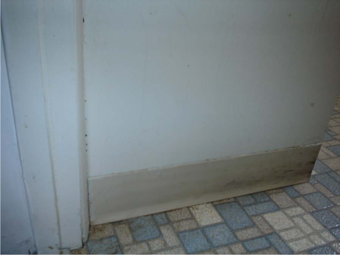
HA # 16 – Non asbestos containing 4” white cove molding and associated mastic
