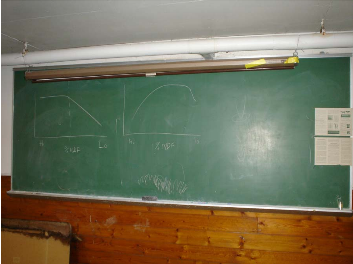
HA #5 – Assumed asbestos containing chalkboards and associated glue pods
