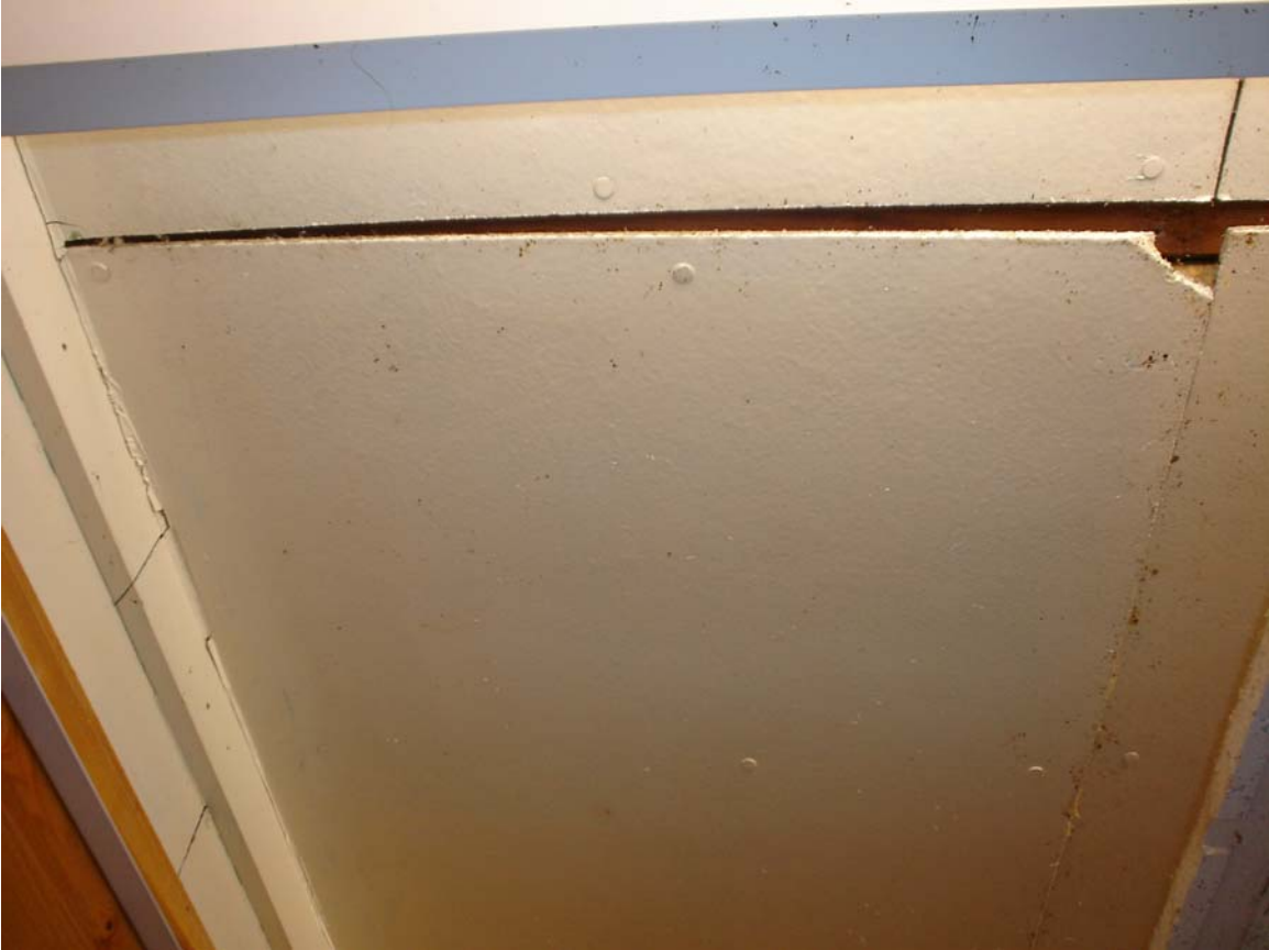
HA #3 – Asbestos containing transite wall and ceiling panels
