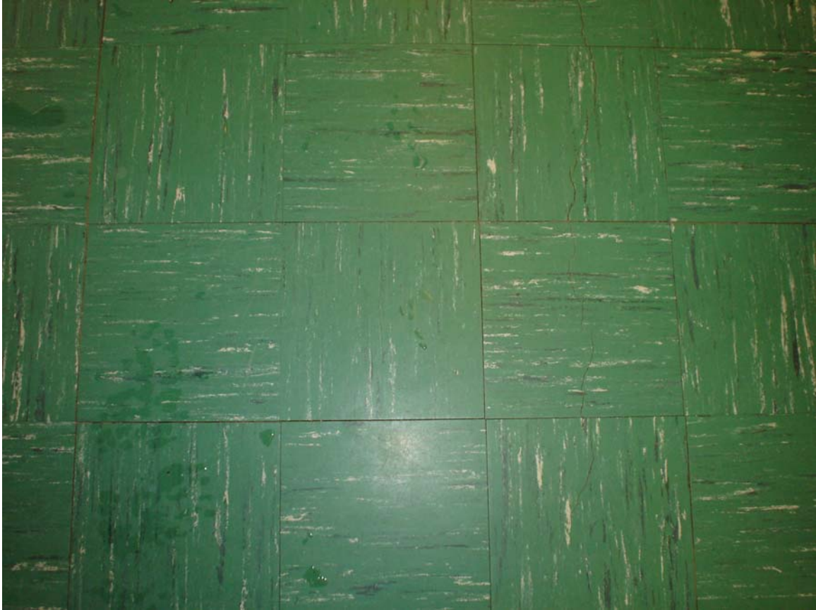
HA #1 – Non asbestos containing 9” x 9” green floor tile with white and black streaks and associated mastic
