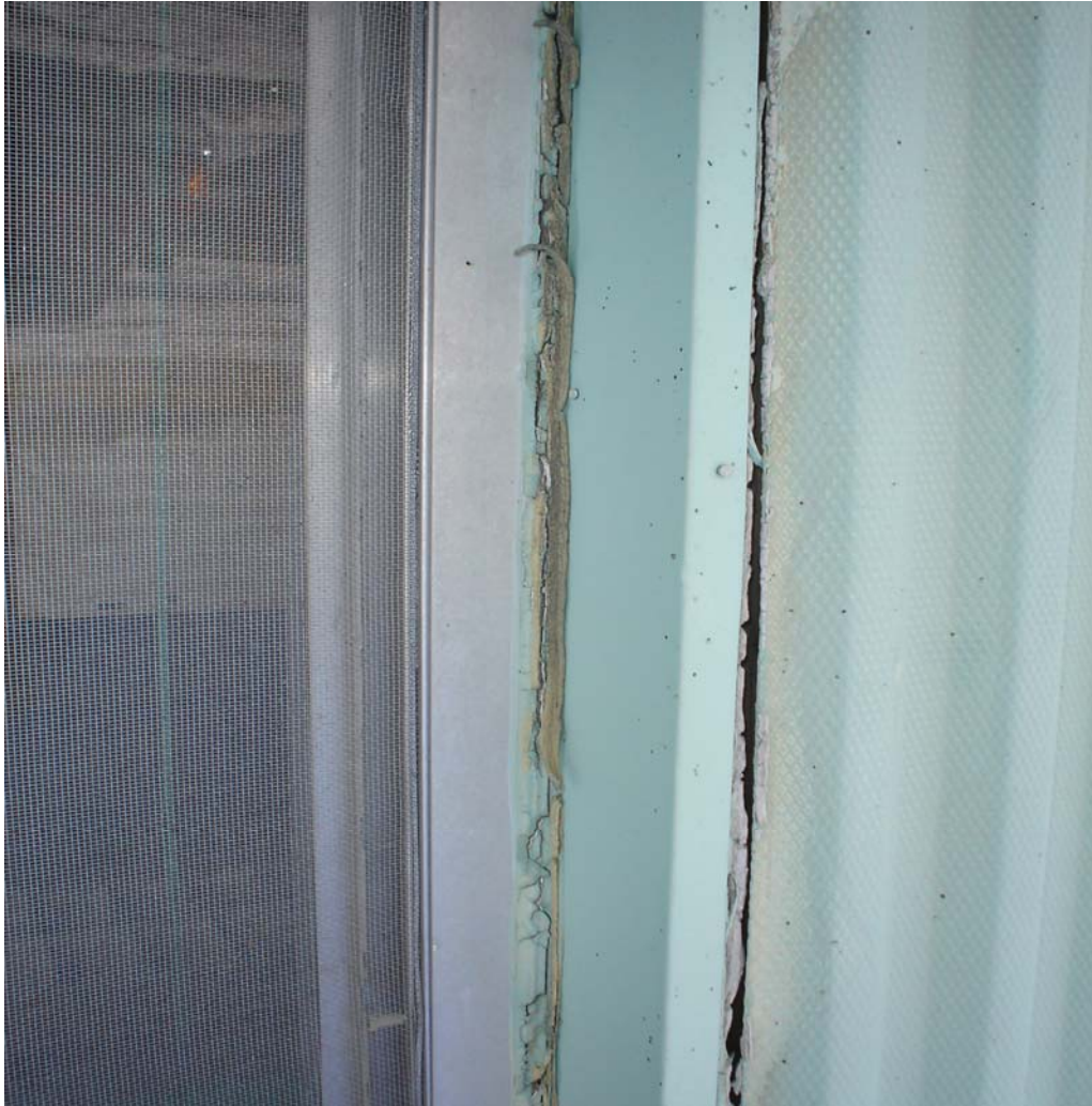
HA # 17 – Asbestos containing window and door frame caulk compound
