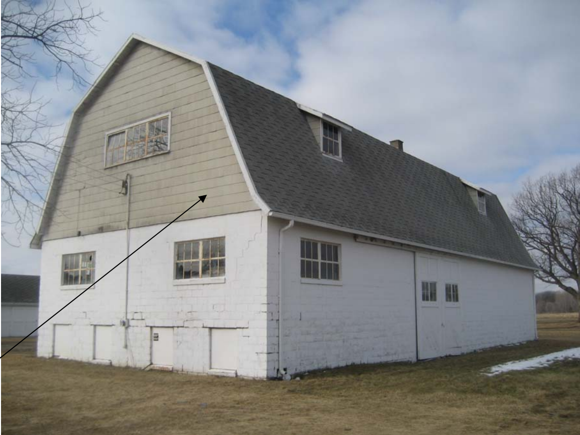
HA #13 – Asbestos containing brown transite siding panels
