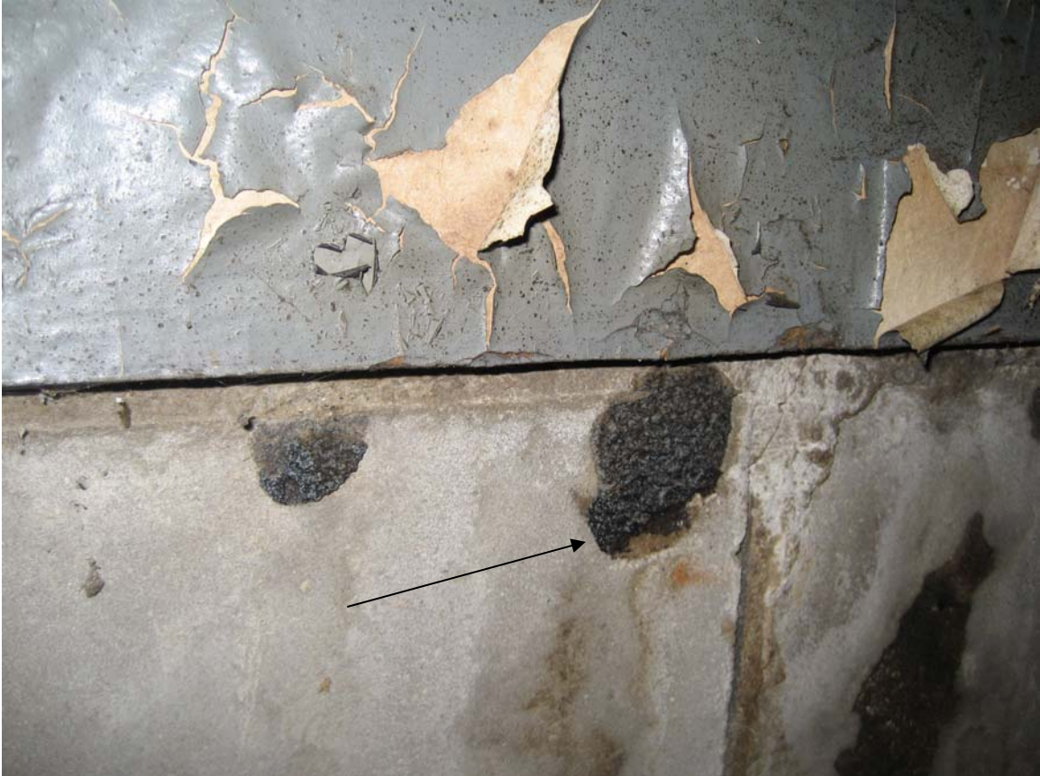
HA #3 – Asbestos containing brown wallboard gluepod
