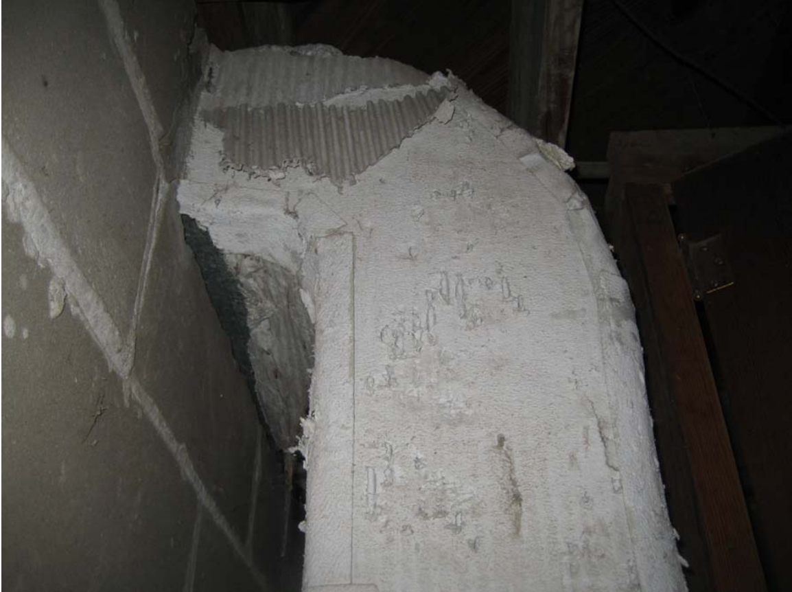
HA #9 – Asbestos containing white duct wrap
