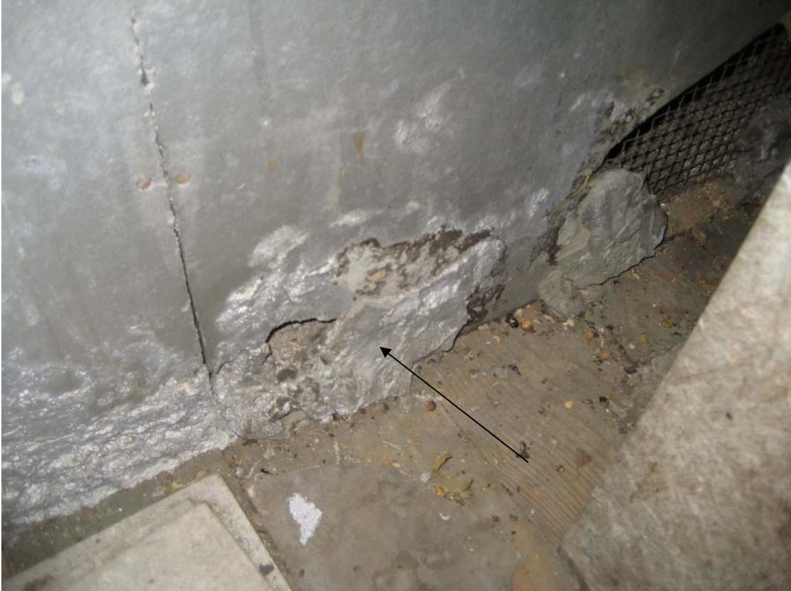
HA #8 – Asbestos containing plaster patch compound
