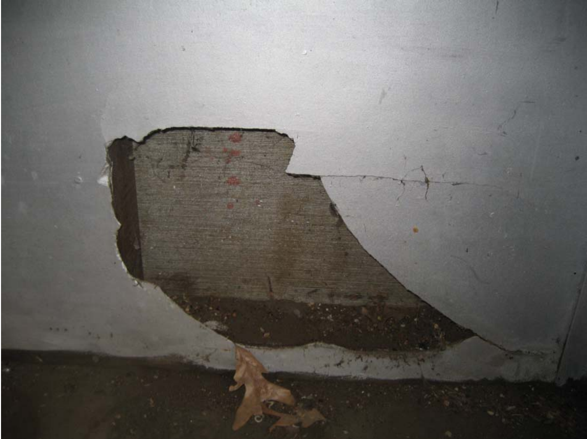
HA #4 – Asbestos containing transite wall board
