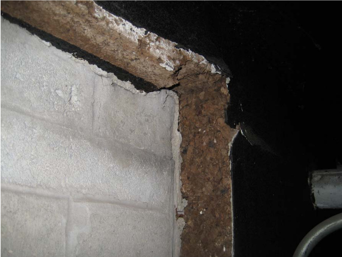
HA #11 – Asbestos containing black tar on brown insulation
