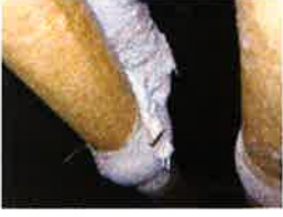
Picture #6--West Wing Room G-29 Basement
