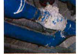
Picture #10--East Wing Mechanical Room G Base...
