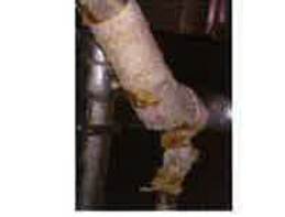
Picture #14--Central Section Mechanical Room D & B-2...
