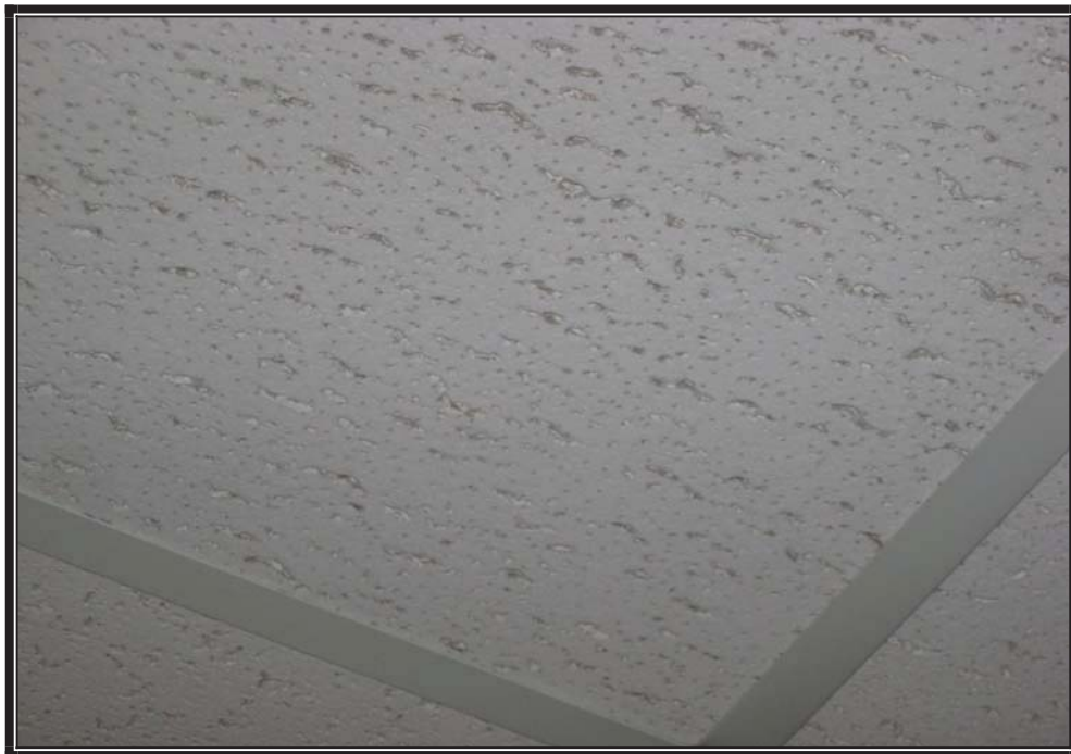
HA-13 2' x 4' Ceiling tile - pinholes and linear fissures
