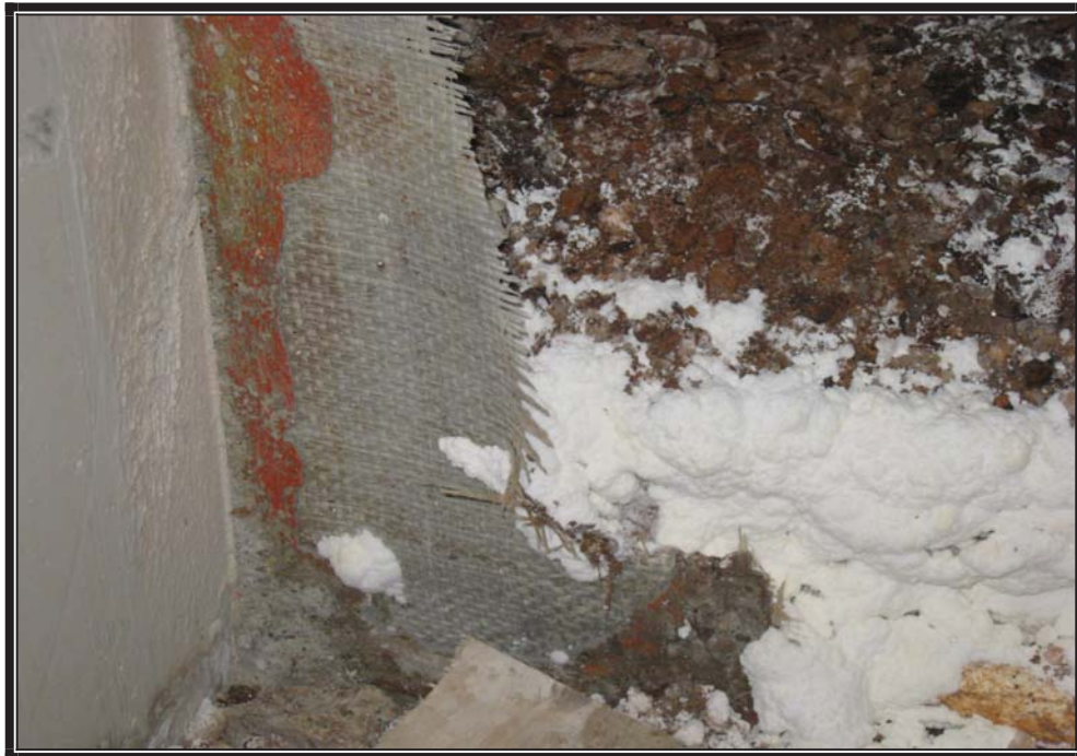
HA-6 Old brine tank lining
