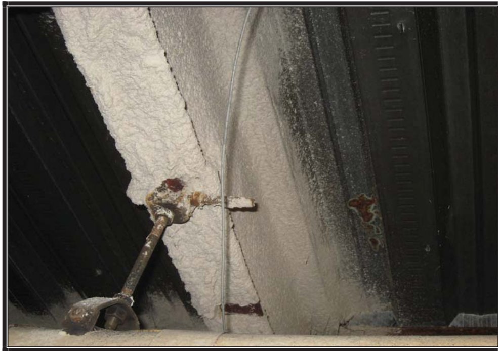
HA-1 Spray-on fire proofing on structural steel
