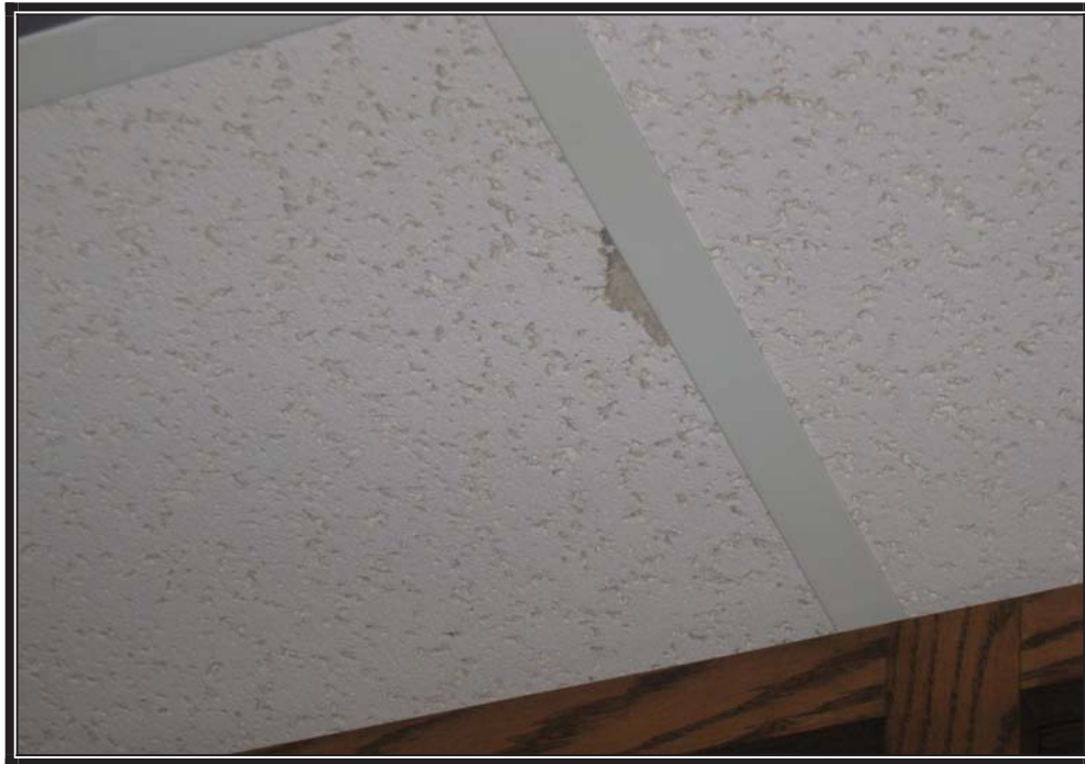
HA-12 2' x 4' Ceiling tile - pinholes and random fissures
