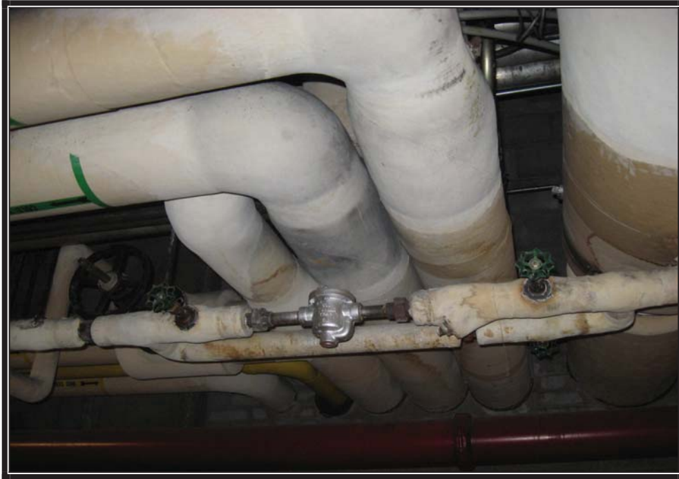
HA-3 Muddied fittings on fiberglass lines <12"
