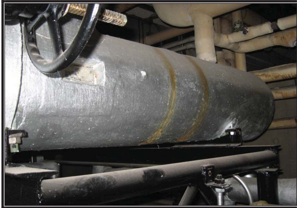
HA-5 Tank insulation
