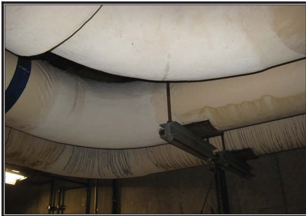
HA-2 Muddled fittings on fiberglass lines >12"
