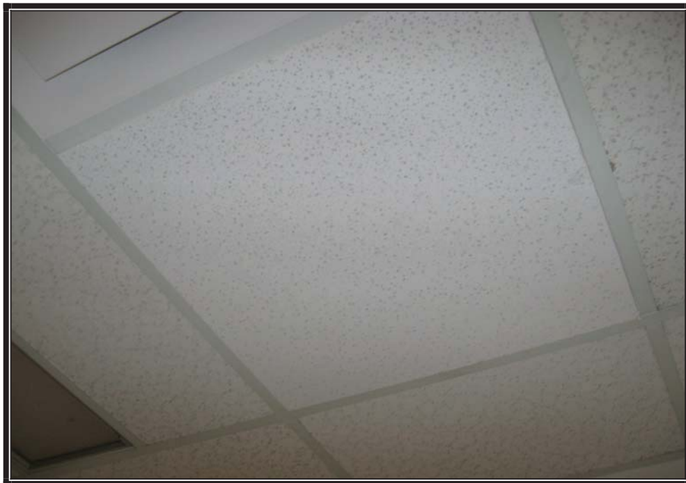
HA-15 2' x 2' Ceiling tile – pinholes and fissures
