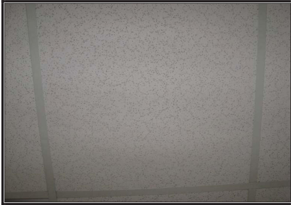
HA-29 2' x 2' Ceiling tile - random sized pinholes with fissures
