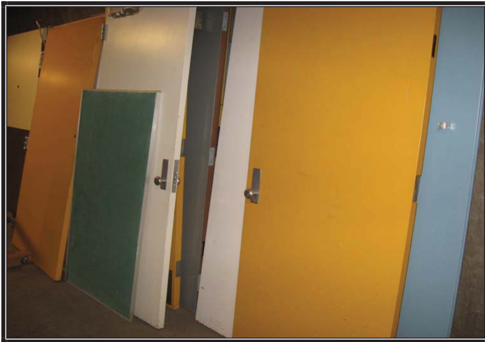
HA-4 Fire doors
