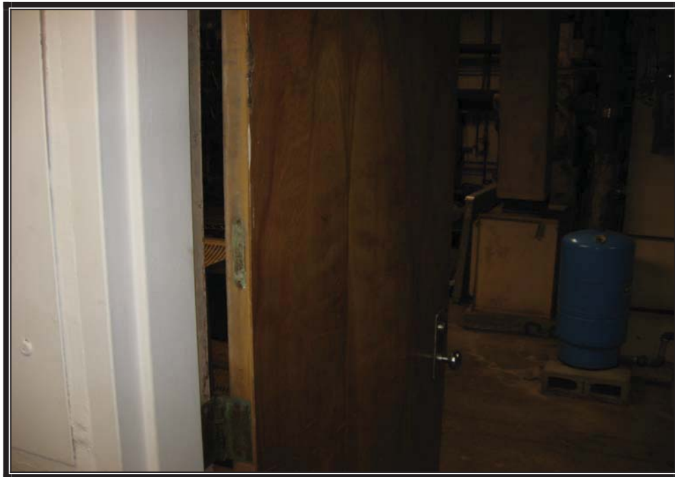
HA6 – Fire Doors
