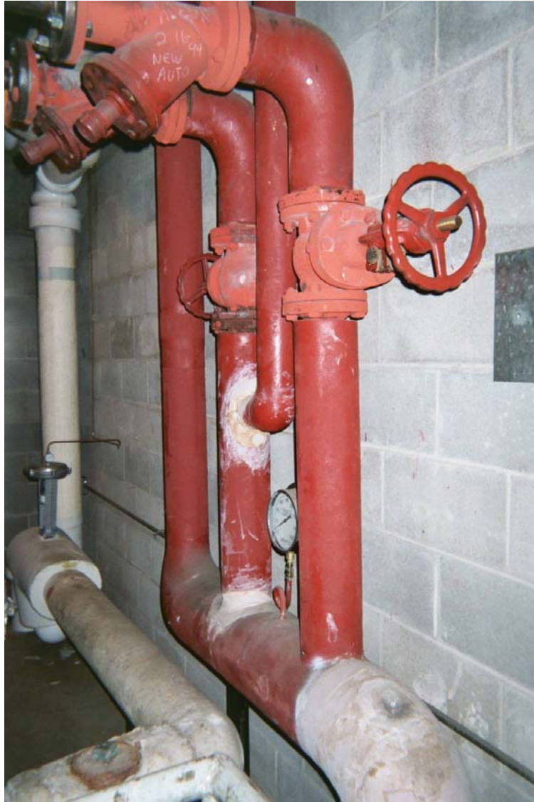
Photo 3 – Asbestos-containing steam/condensate pipe straight insulation
