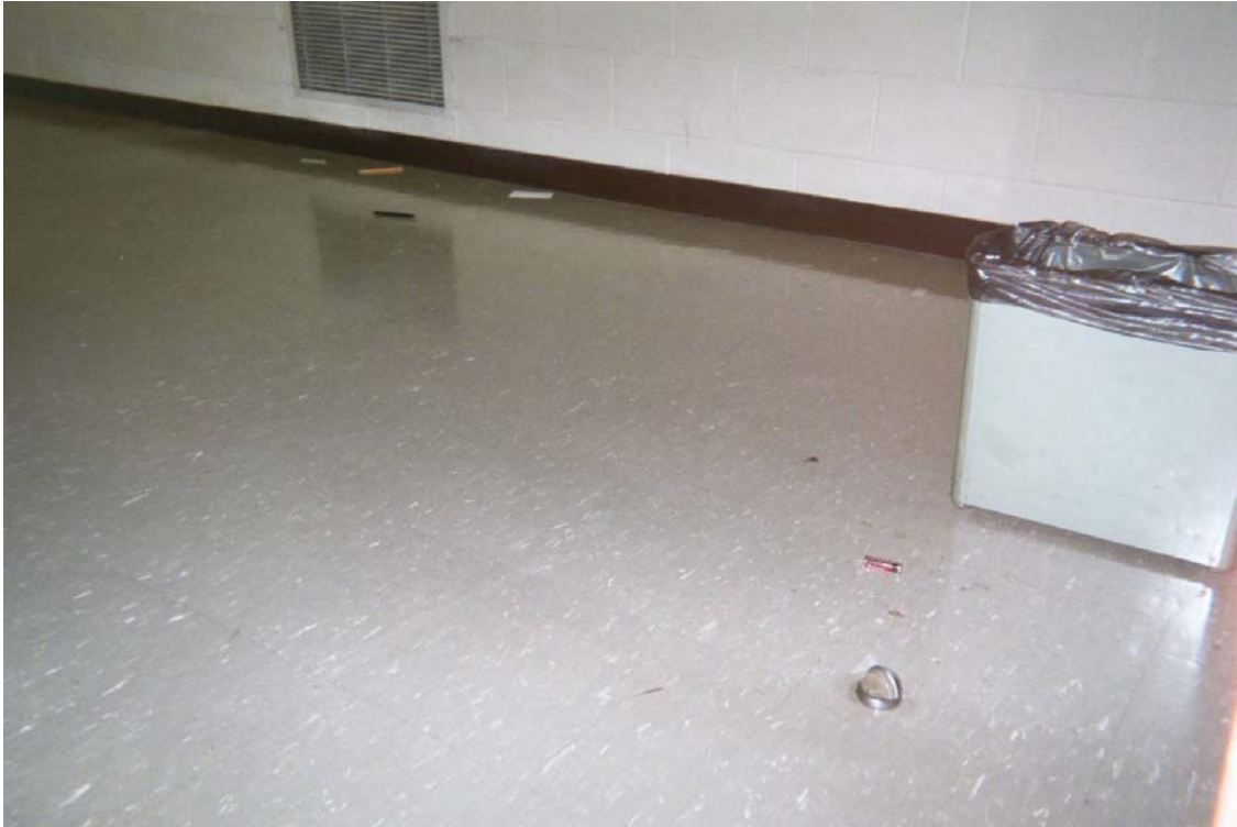
Photo 17 – Asbestos-containing 12” x 12” gray floor tile with white streaks and associated mastic
