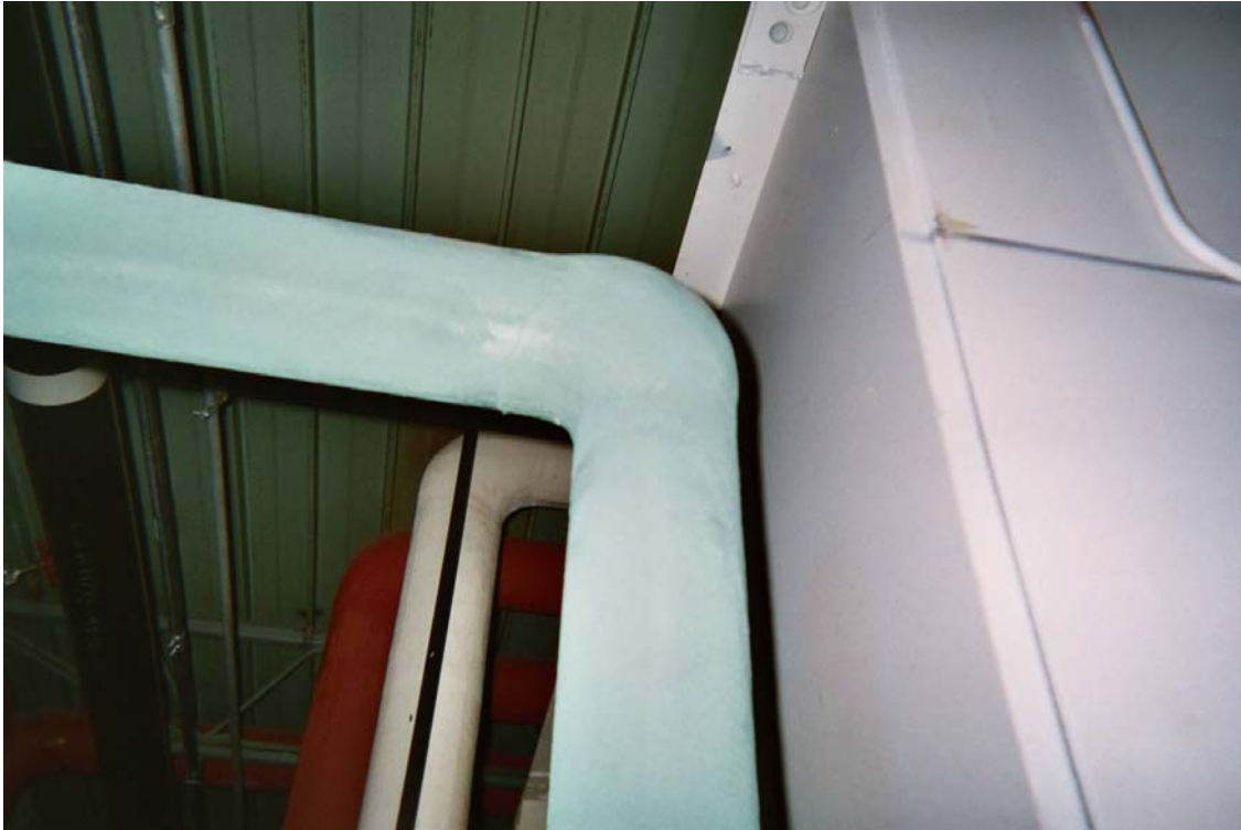
Photo 2 – Asbestos-containing domestic water pipe joint insulation
