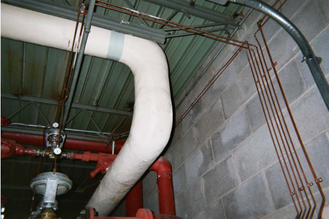
Photo 5 – Asbestos-containing chilled water pipe joint insulation
