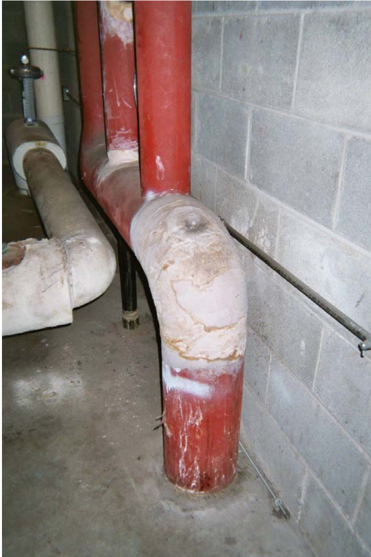
Photo 4 – Asbestos-containing steam/condensate pipe joint insulation
