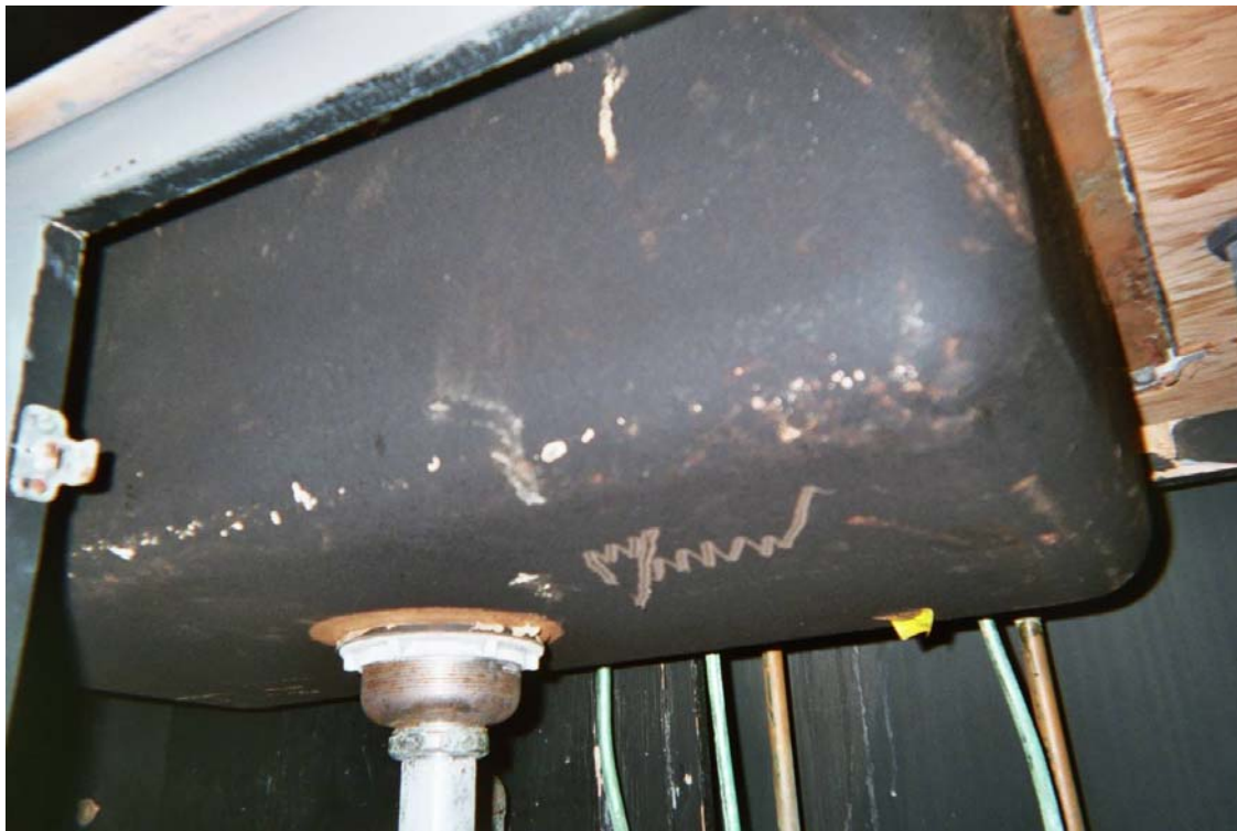
Photo 11 – Asbestos-containing black sink undercoating
