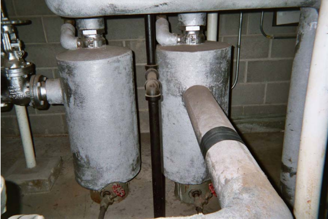
Photo 6 – Asbestos-containing radiation heat tank insulation
