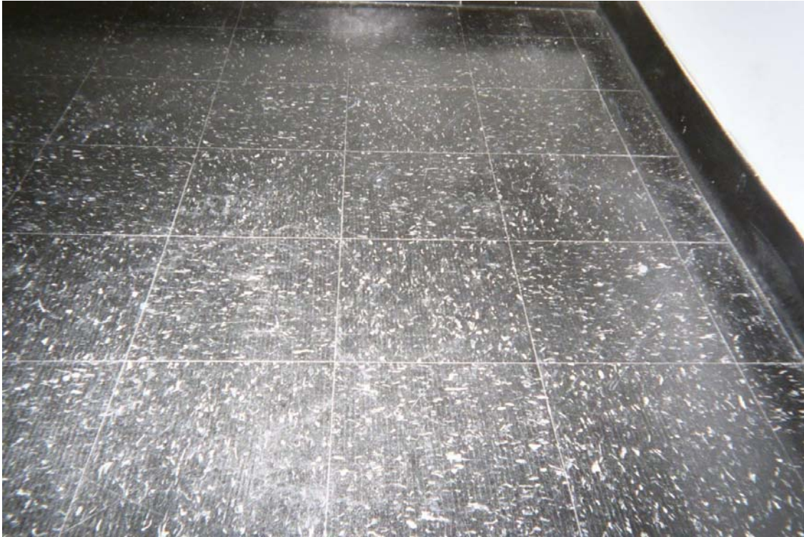
Photo 8 – Asbestos-containing 9” x 9” black floor tile with white specks and associated mastic
