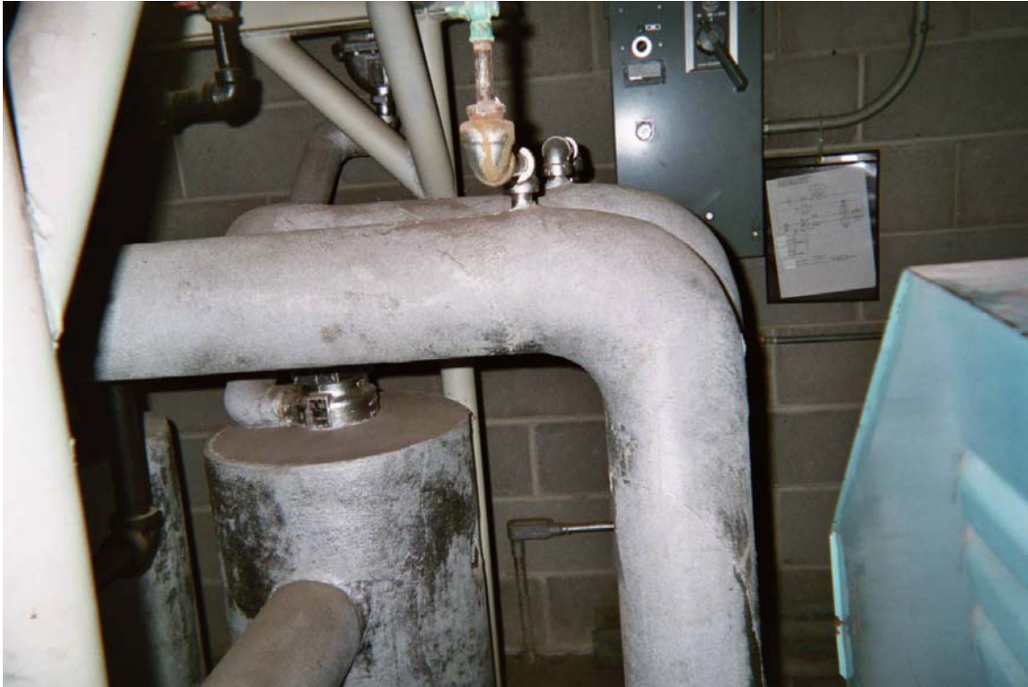
Photo 7 – Asbestos-containing radiation heat pipe joint insulation
