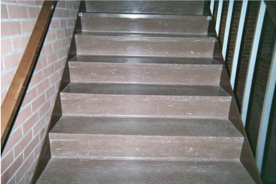
Photo 14 – Asbestos-containing brown vinyl stair tread
