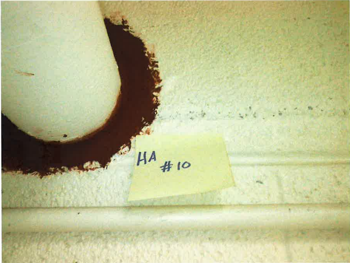
HA #10 – Non asbestos-containing red firestop caulk
