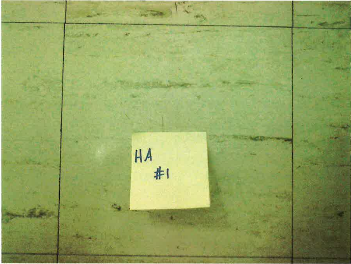
HA #1 – Non asbestos-containing 9" x 9" gray floor tile with dark green streaks and associated mastic
