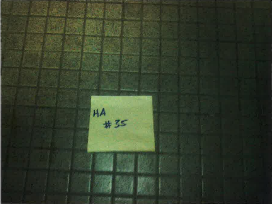
HA #35 – Non asbestos-containing 1/2" x 1/2" gray ceramic floor tile with black specks bedding compound and grout
