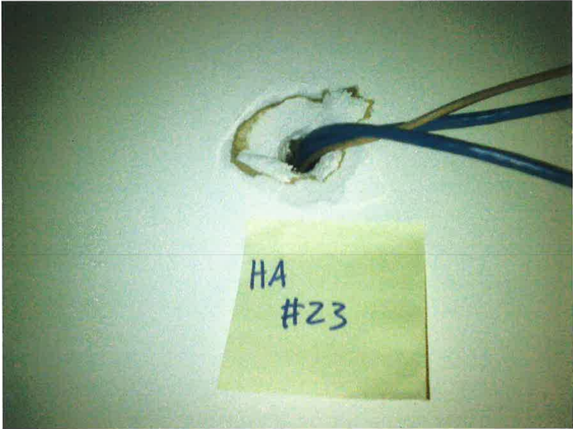
HA #23 – Non asbestos-containing fire-rated drywall
