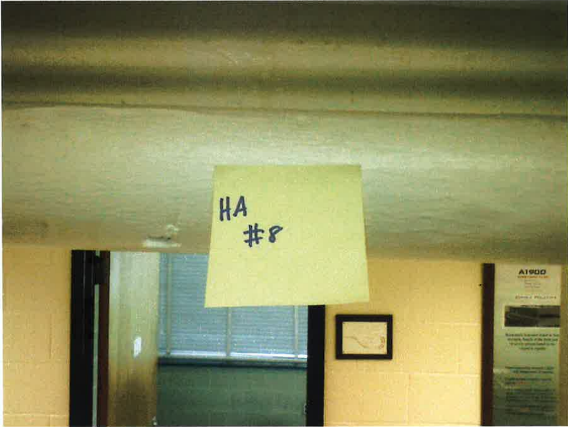
HA #8 – Non asbestos-containing steam and condensate pipe straight insulation (wrap on fiberglass line)
