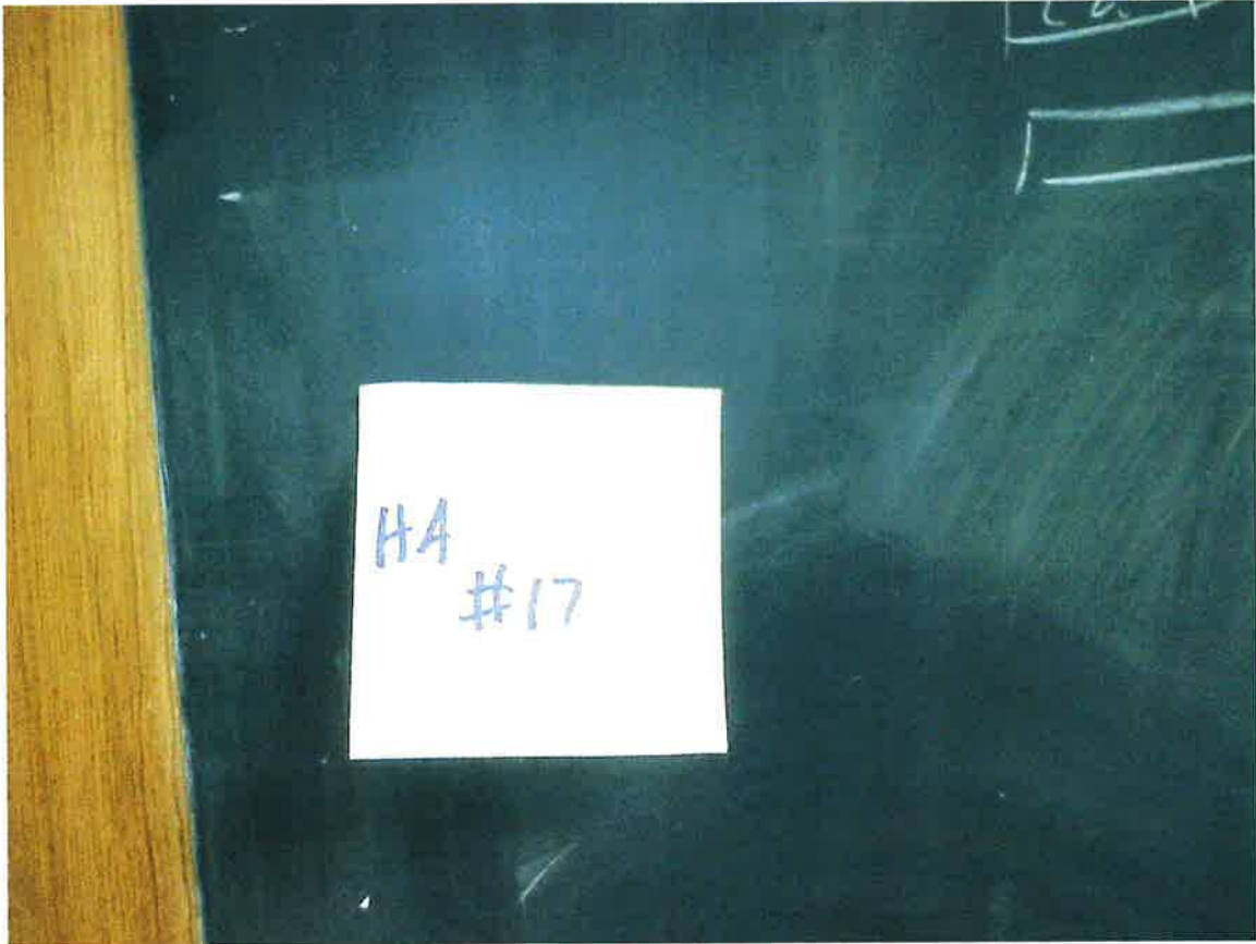
HA #17 – Assumed asbestos-containing black chalkboard
