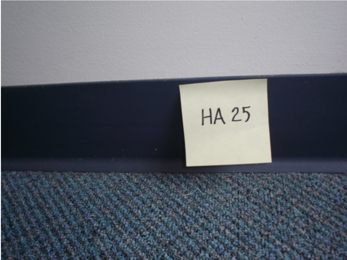
HA #25 – Non asbestos-containing 4" blue/gray cove molding and associated mastic
