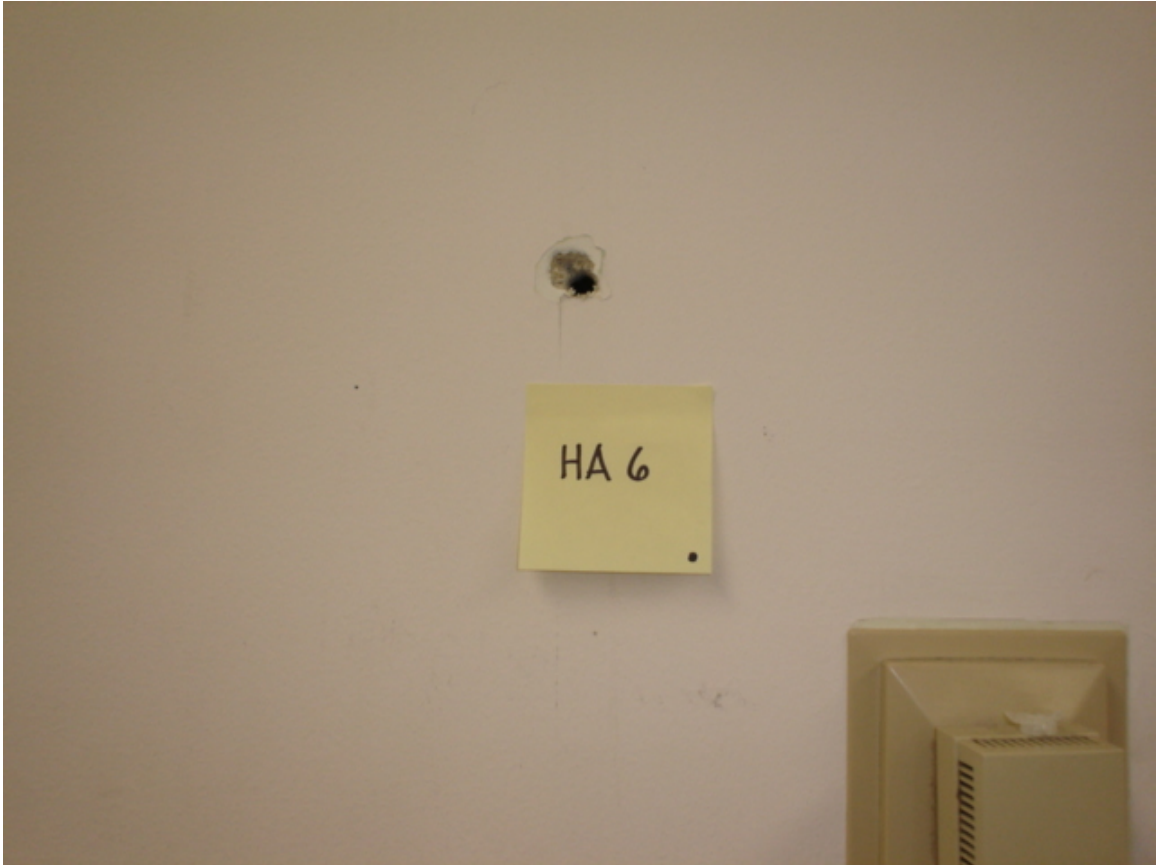
HA #6 – Non asbestos-containing plaster
