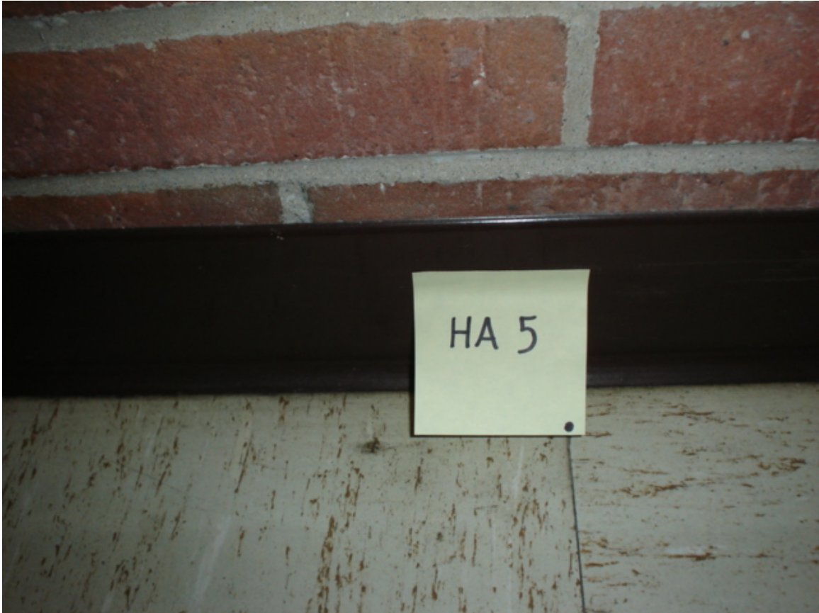
HA #5 – Non asbestos-containing 4" brown cove molding and associated mastic
