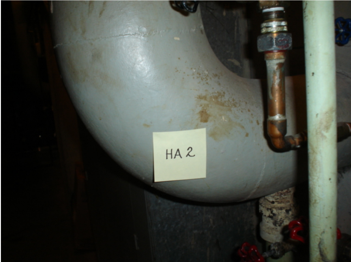
HA #2 – Asbestos-containing steam/condensate supply and return pipe joint and hanger insulation
