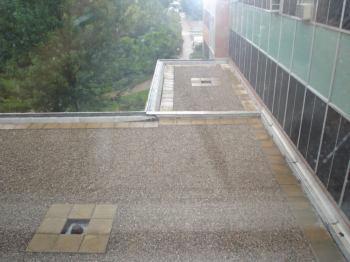
HA #49 – Assumed asbestos-containing roofing materials and products
