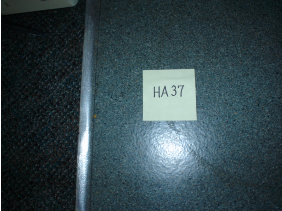
HA #37 – Non asbestos-containing cream vinyl flooring with black and cream specks and associated mastic
