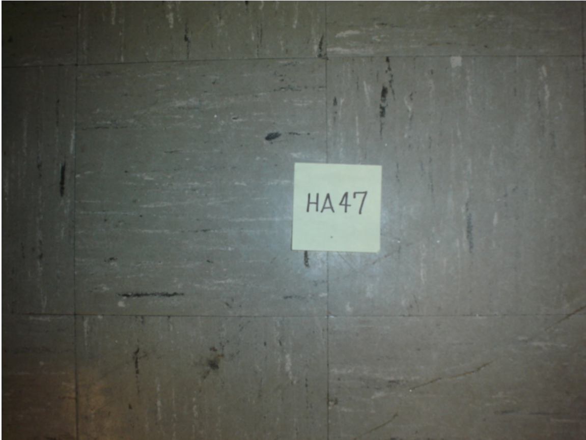
HA #47 – Asbestos-containing 9" x 9" light gray floor tile with black and cream streaks and associated non asbestos-containing mastic
