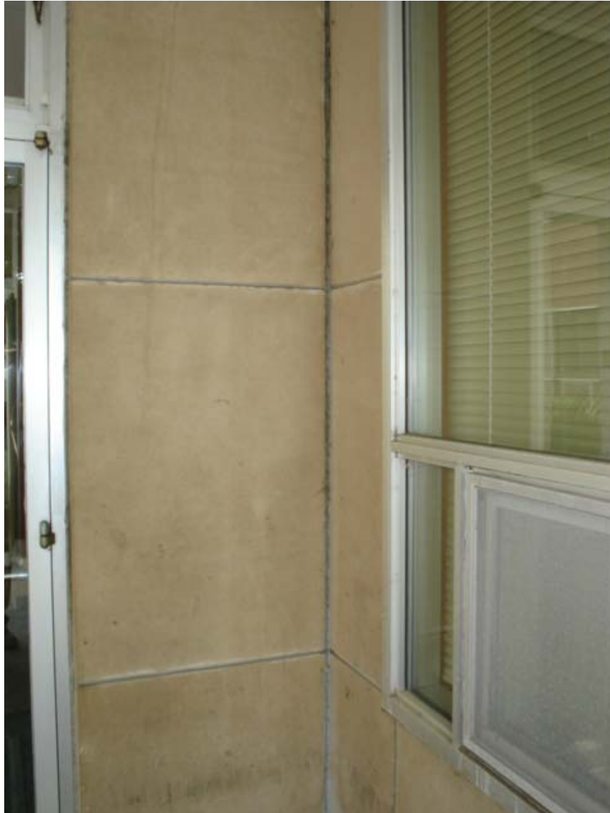
HA #29 – Assumed asbestos-containing window and door frame caulk compound
