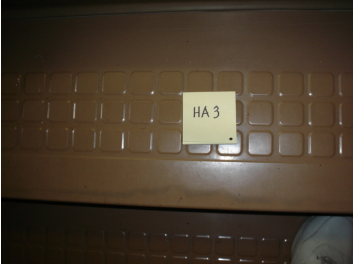
HA #3 – Non asbestos-containing tan vinyl stair tread and flooring with small squares and associated mastic
