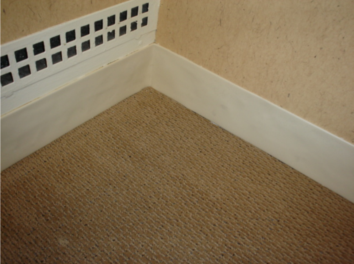
HA #52 – Non asbestos-containing 4" cream cove molding and associated mastic
