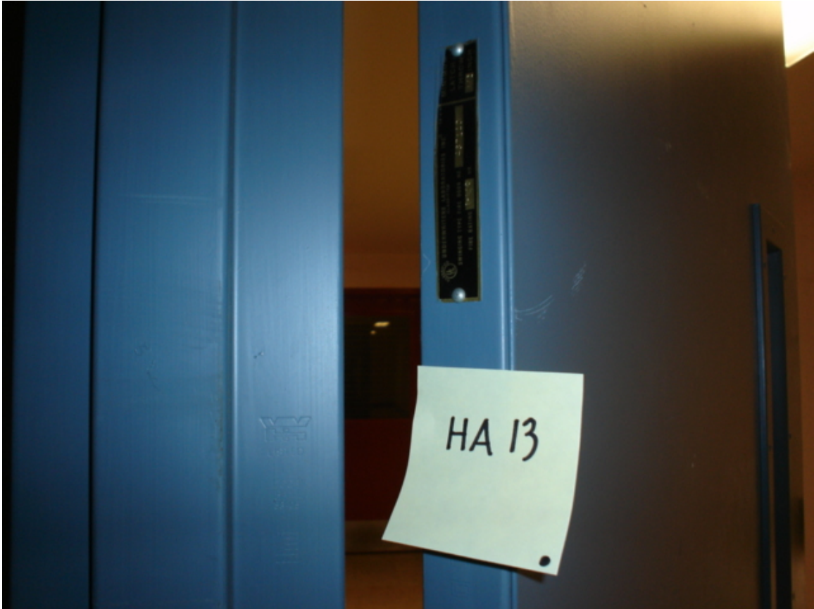
HA #13 – Assumed asbestos-containing fire door and frame
