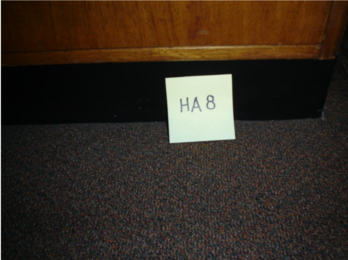
HA #8 – Non asbestos-containing 4" black cove molding and associated mastic
