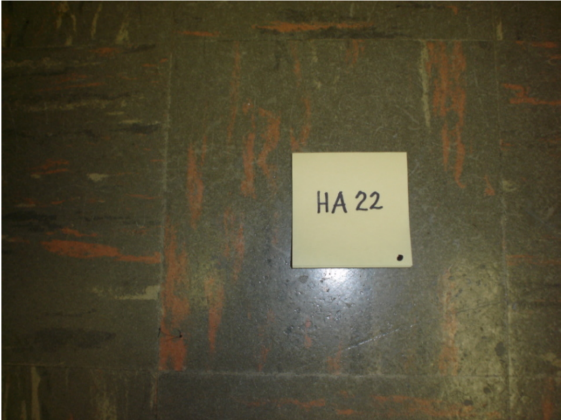
HA #22 – Asbestos-containing 9" x 9" gray floor tile with pink, cream and gray streaks and associated non asbestos-containing mastic
