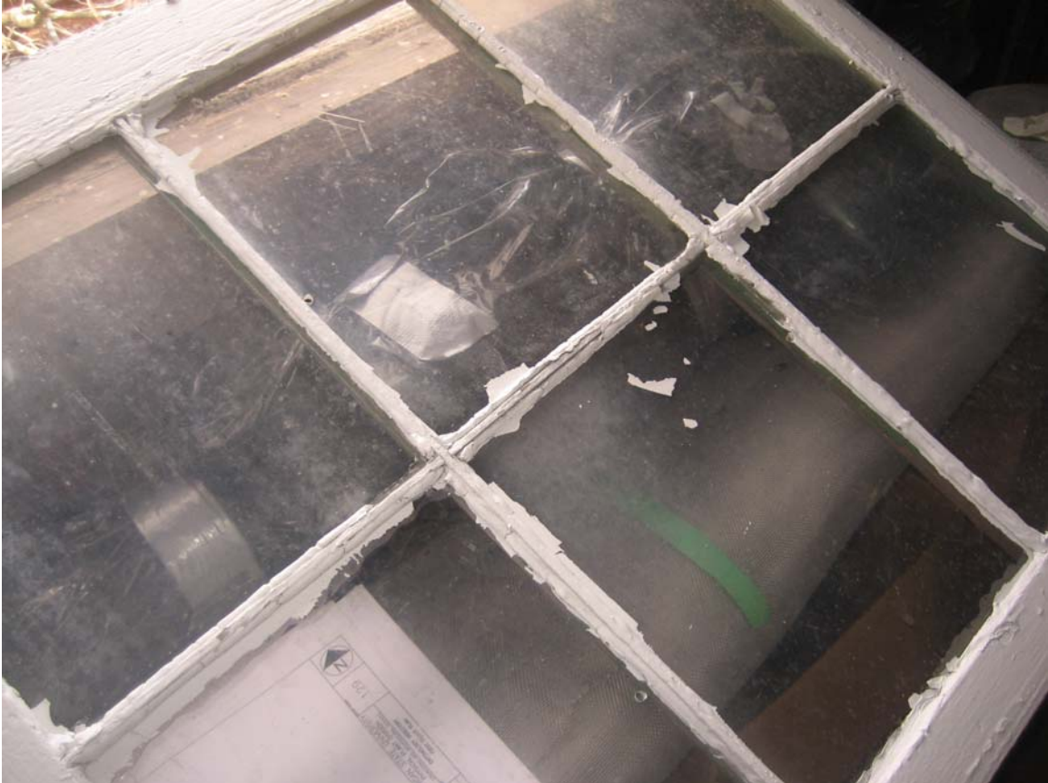
HA #1 – Asbestos containing white to gray window glazing
