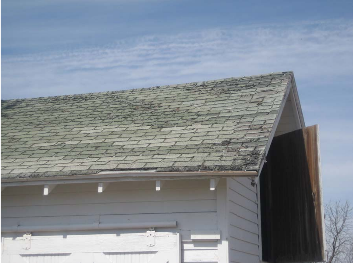
HA #2 – Assumed asbestos containing roofing materials and products
