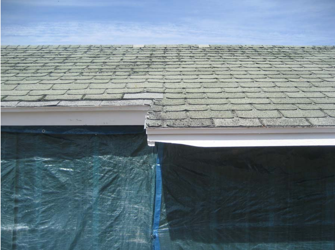
HA #1 – Assumed asbestos containing roofing materials and products
