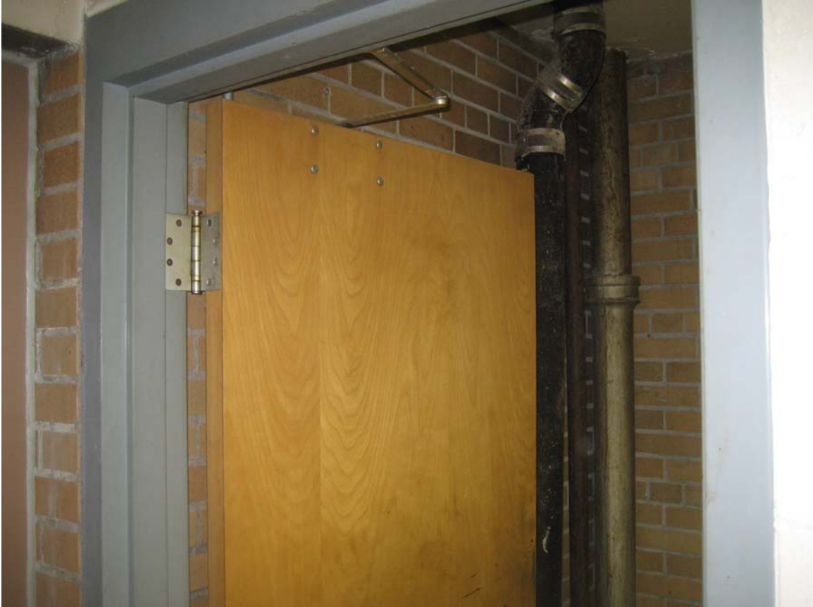
HA #3 – Assumed asbestos containing fire door and frame
