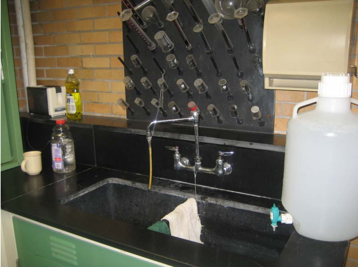
HA #1 – Assumed asbestos containing lab bench, sink, and drying rack
