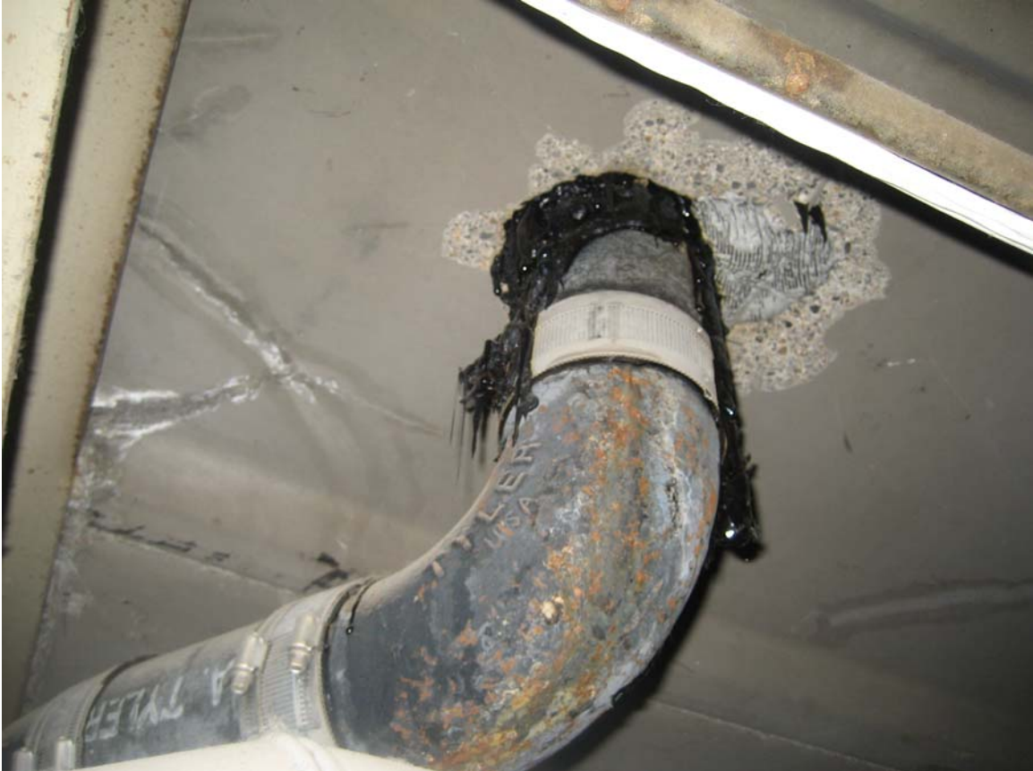
HA #5 – Asbestos containing black roof tar
