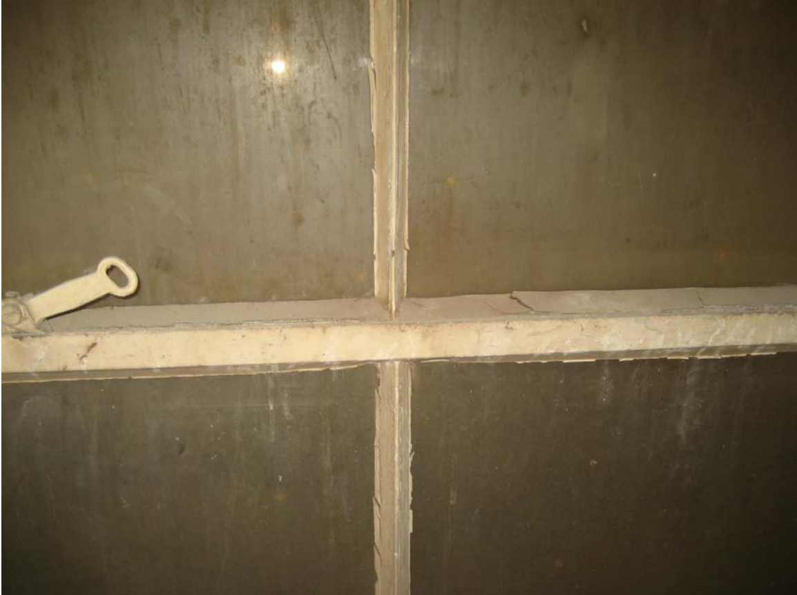
HA #4 – Asbestos containing brown window glazing
