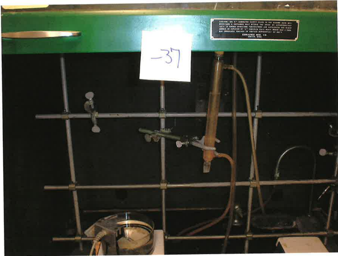
HA #37 – Assumed asbestos containing transite fume hood
