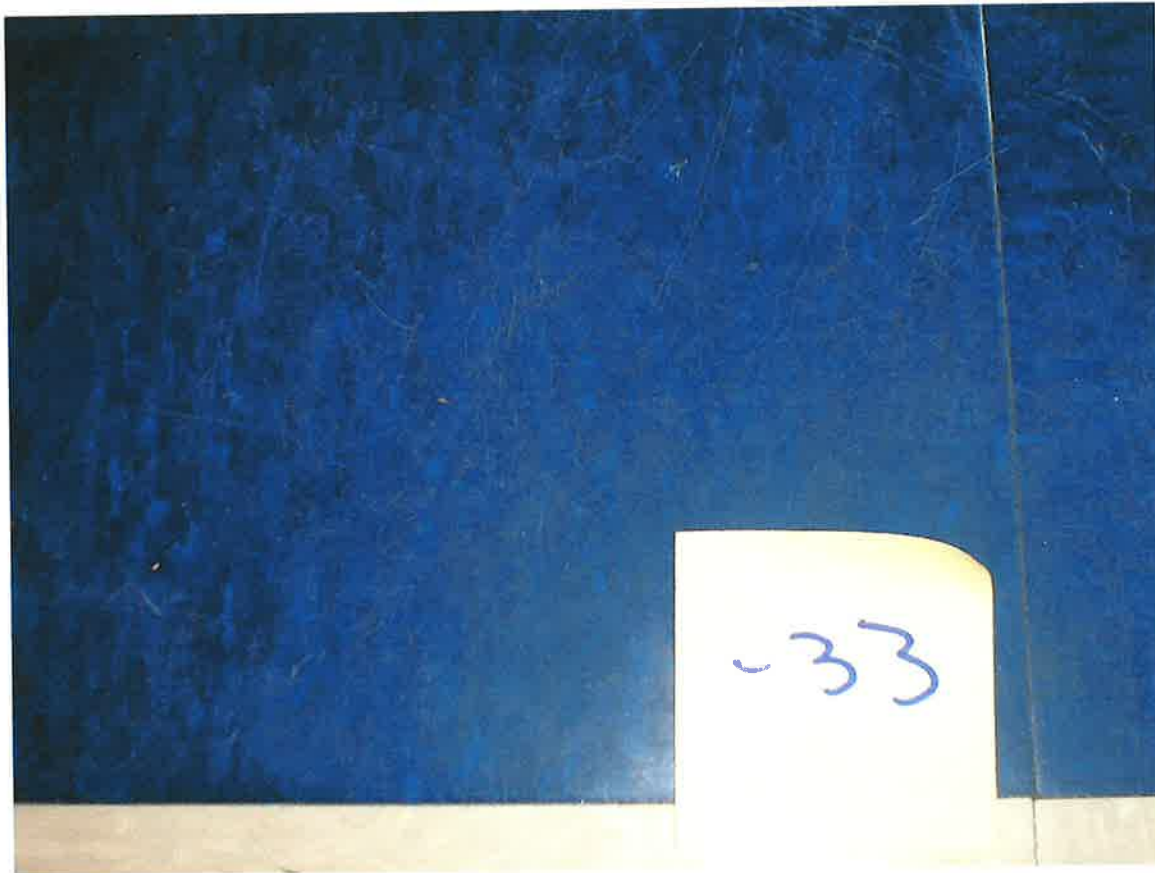
HA #33 – Non asbestos containing 12" x 12" blue floor tile with marble pattern and asbestos containing associated mastic
