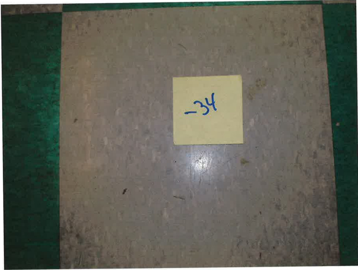
HA #34 – Non asbestos containing 12” x 12” gray floor tile with marble pattern and associated mastic
