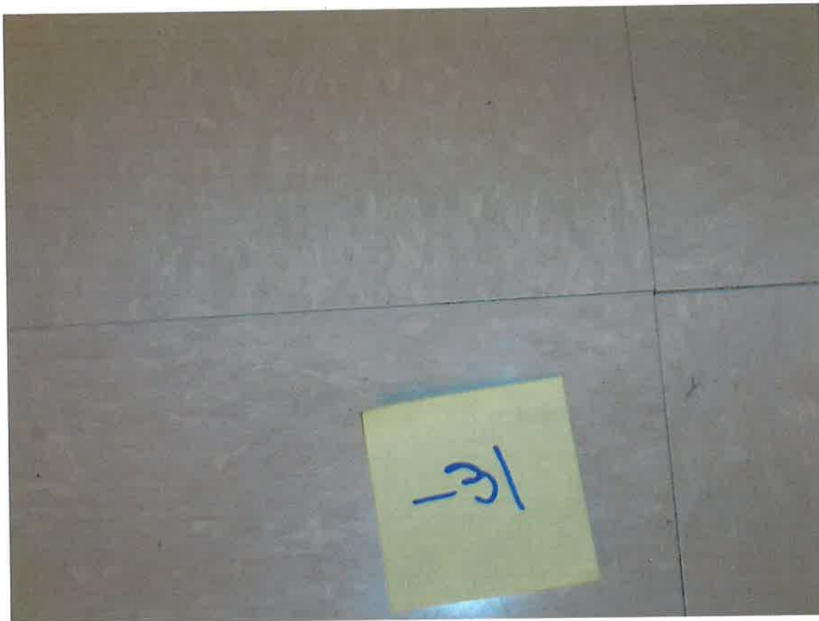
HA #31 – Non asbestos containing 12” x 12” cream floor tile with marble pattern and asbestos containing associated mastic
