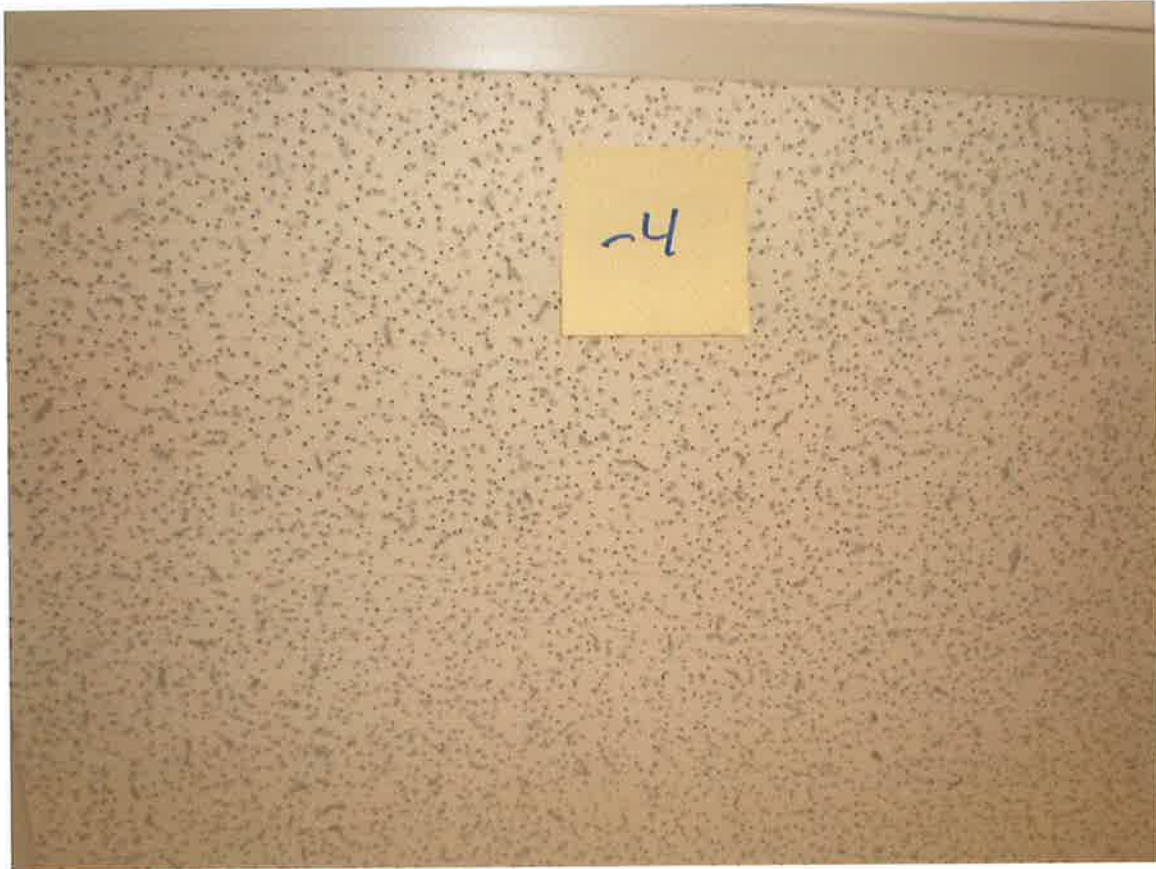
HA #4 – Non asbestos containing 2' x 2' white lay-in ceiling tile with pin holes and fissures
