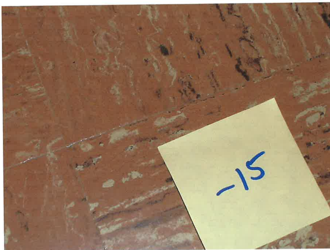
HA #15 – Asbestos containing 9” x 9” light brown floor tile with cream and brown streaks and non asbestos containing associated mastic
