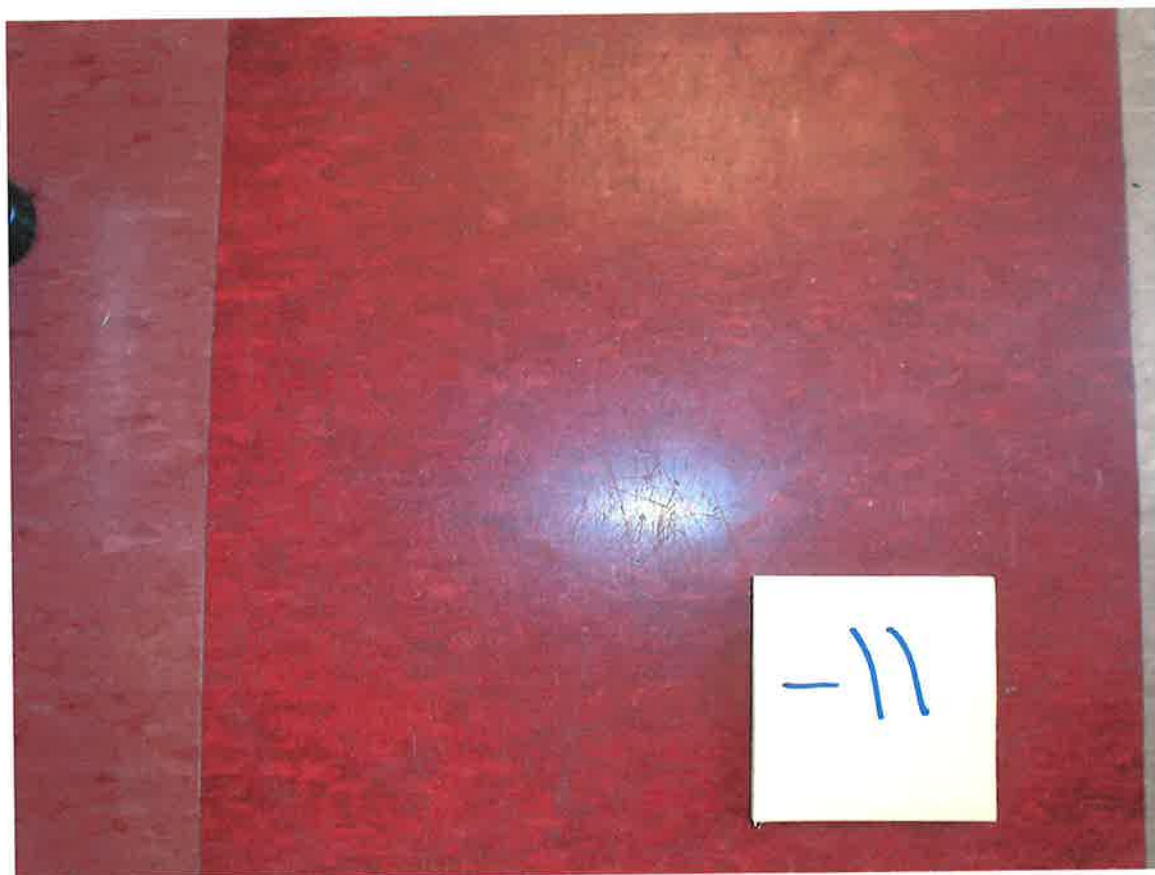
HA #11 – Non asbestos containing 12” x 12” red floor tile with marble pattern and asbestos containing associated mastic
