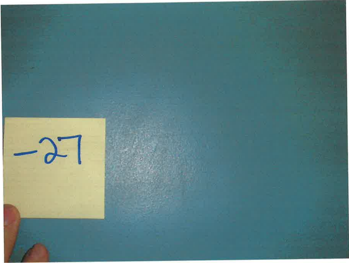
HA #27 – Assumed asbestos containing fire door and frame
