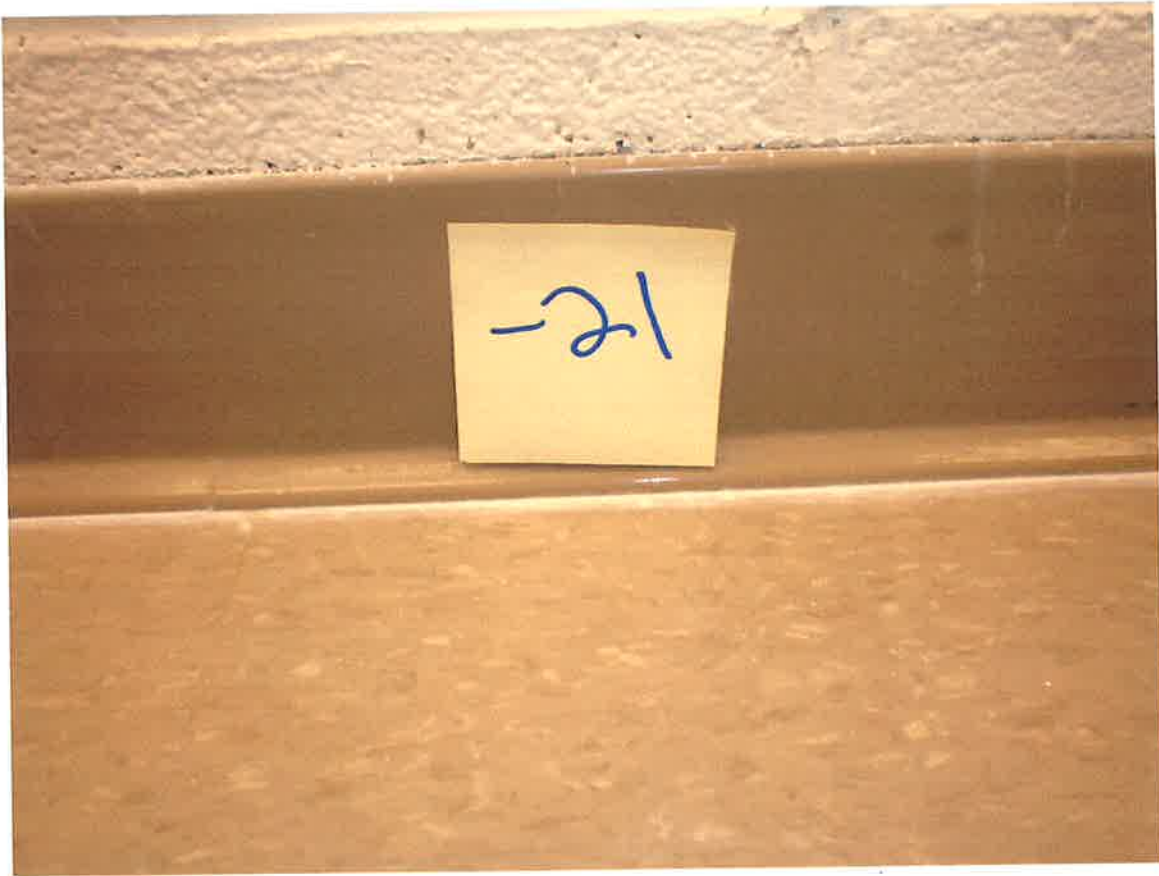
HA #21 – Non asbestos containing 4” beige cove molding and associated mastic
