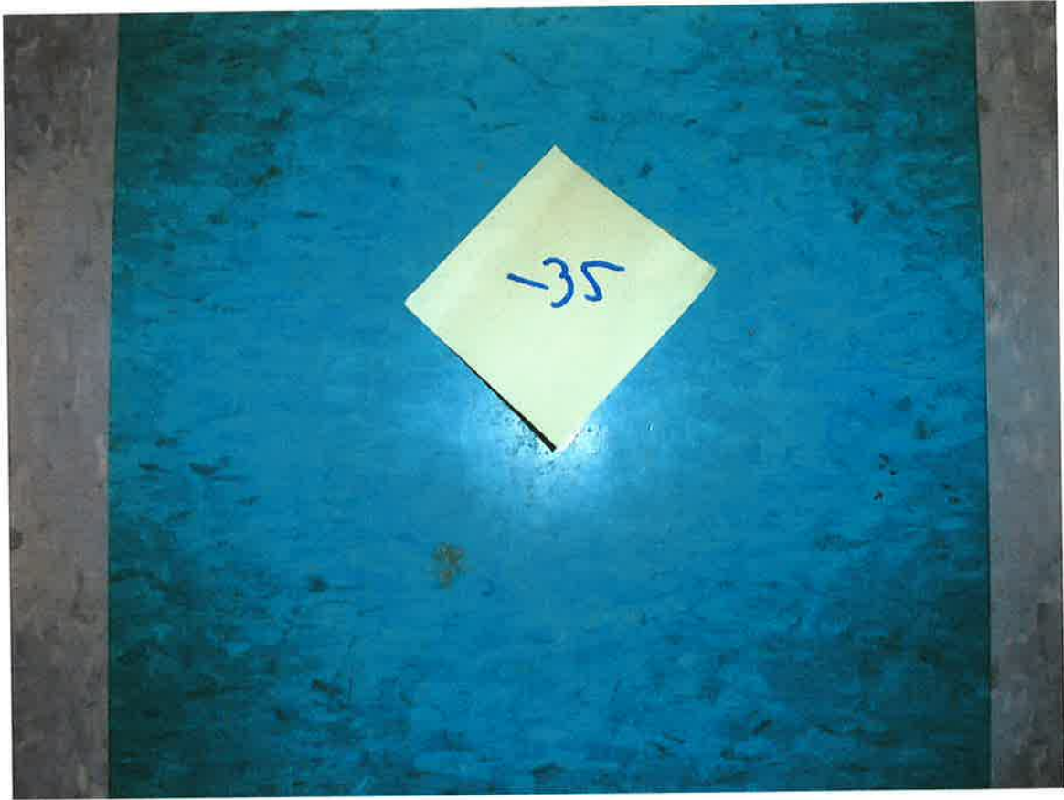
HA #35 – Non asbestos containing 12” x 12” green floor tile with marble pattern and associated mastic
