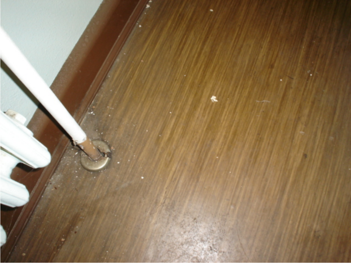
HA #14 – Non asbestos-containing brown linoleum flooring with wood grain pattern and associated backing
