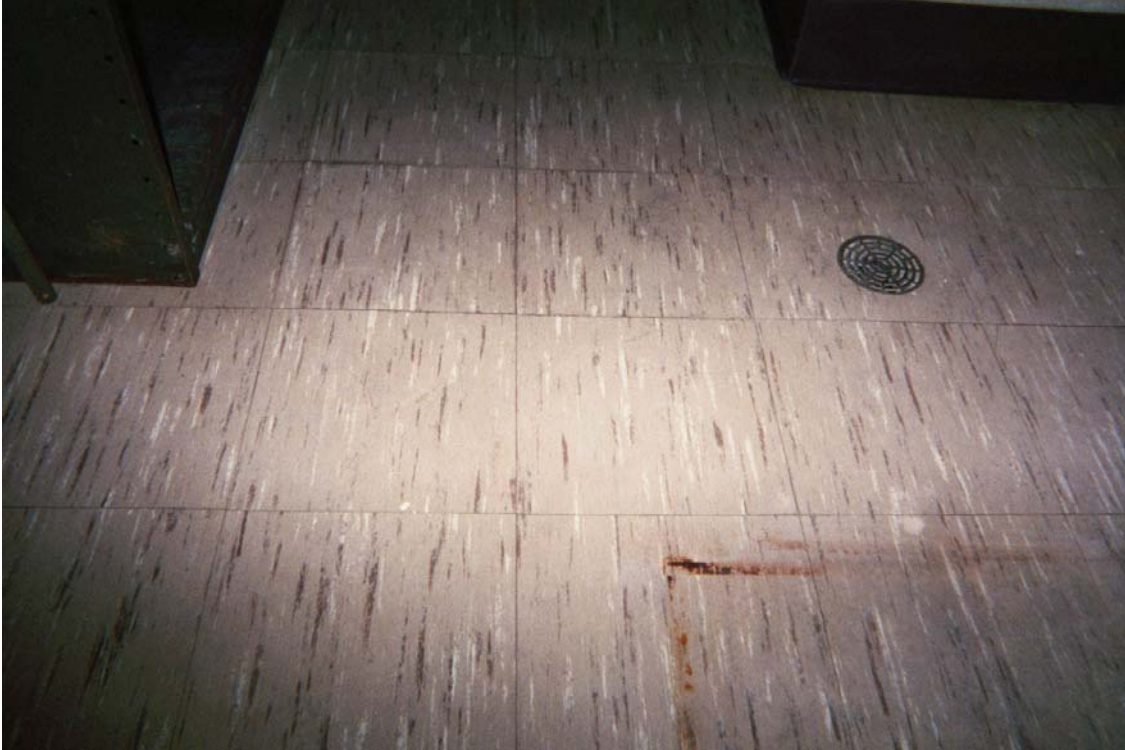
Photo 6 – Asbestos-containing 12” x 12” tan floor tile with cream and brown streaks
