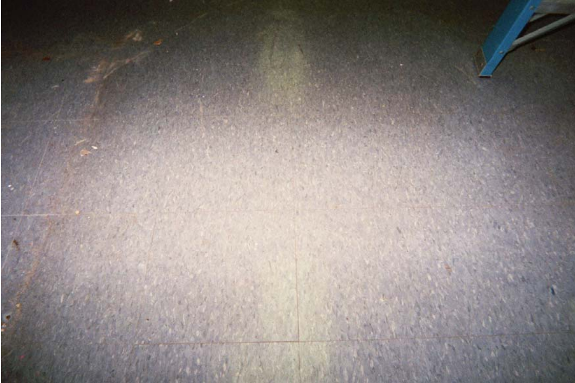
Photo 8 – Asbestos-containing 12” x 12” gray floor tile with marble pattern
