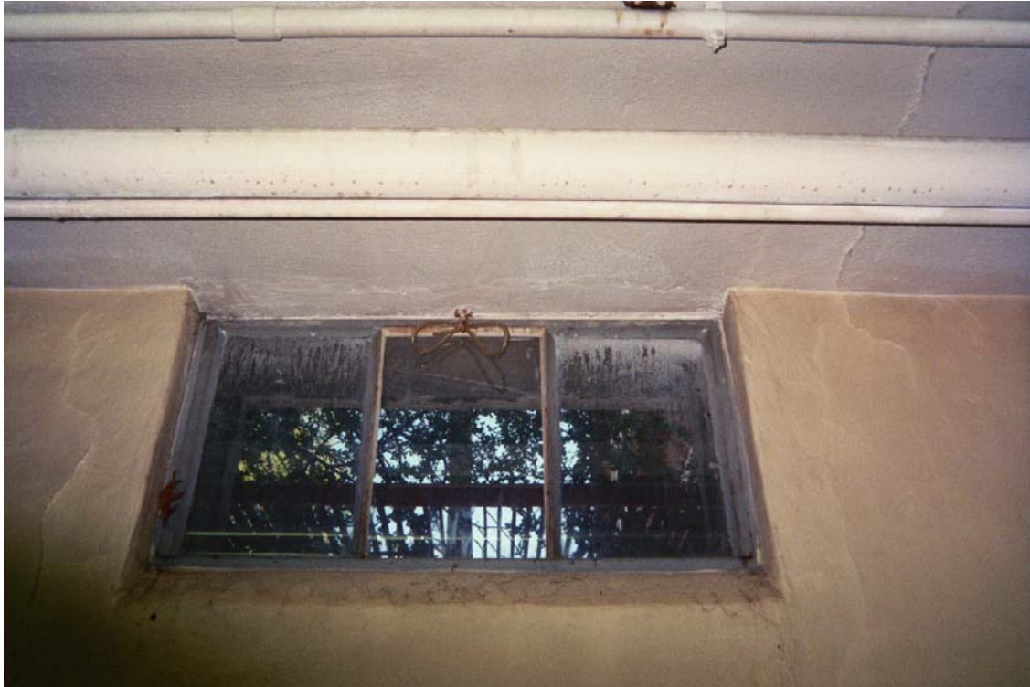
Photo 7 – Assumed asbestos-containing window frame glazing compound
