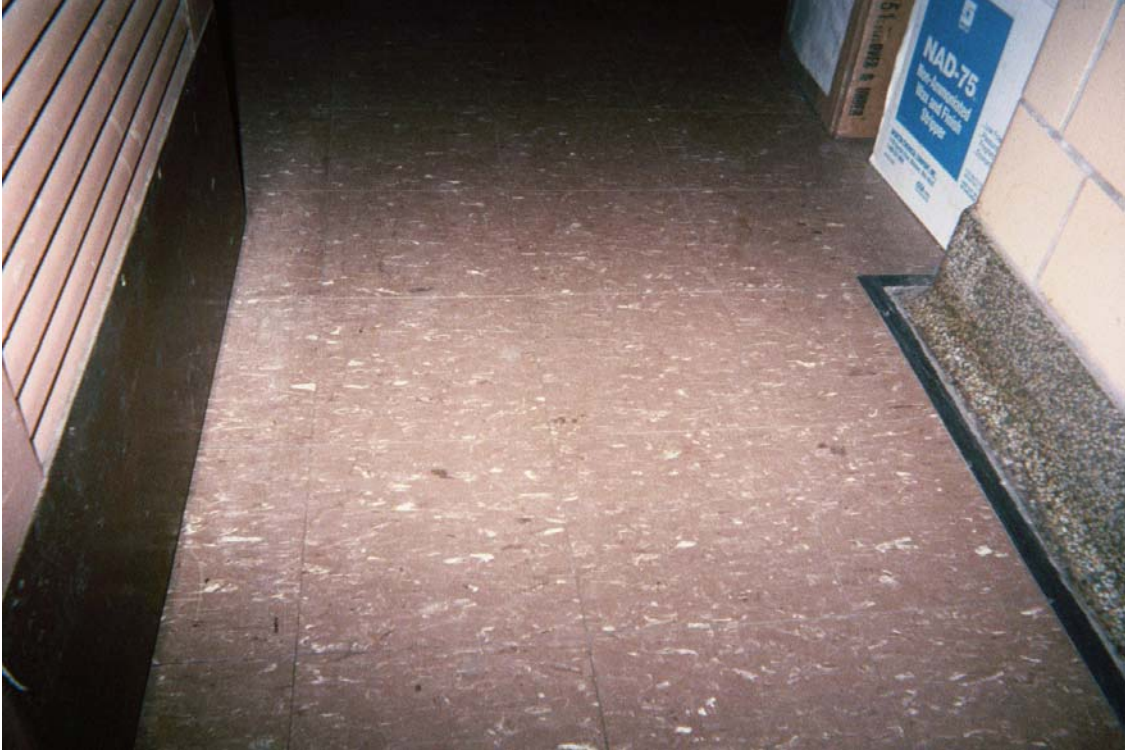
Photo 9 – Asbestos-containing 12” x 12” tan floor tile with cream and brown streaks
