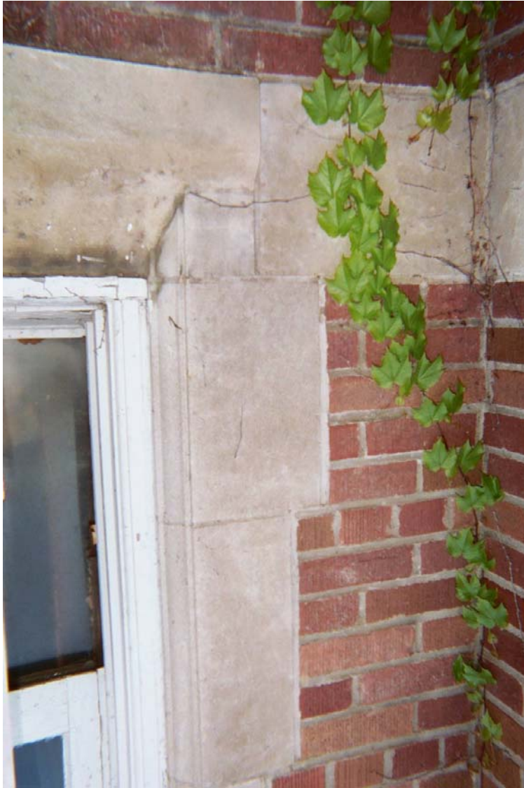
Photo 11 – Assumed asbestos-containing window and door frame caulk compound
