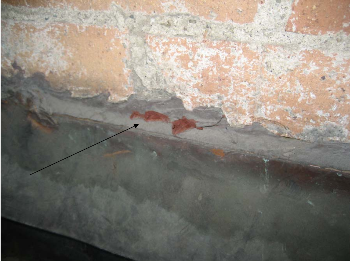
HA #3 – Asbestos containing black and brown building caulk
