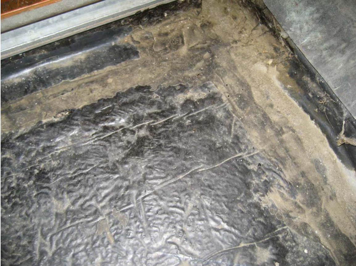
HA #4 – Non asbestos containing black vinyl waterproof material
