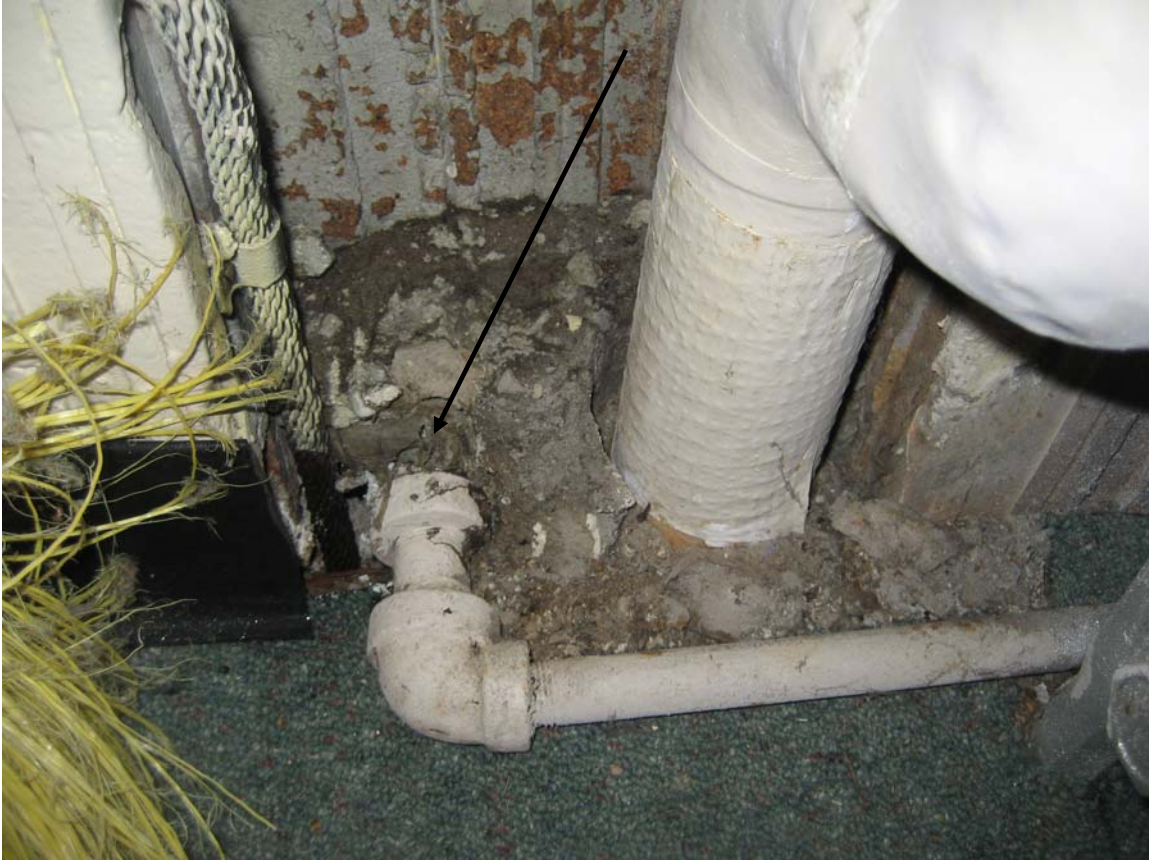
HA #6 – Asbestos containing pipe insulation between floors
