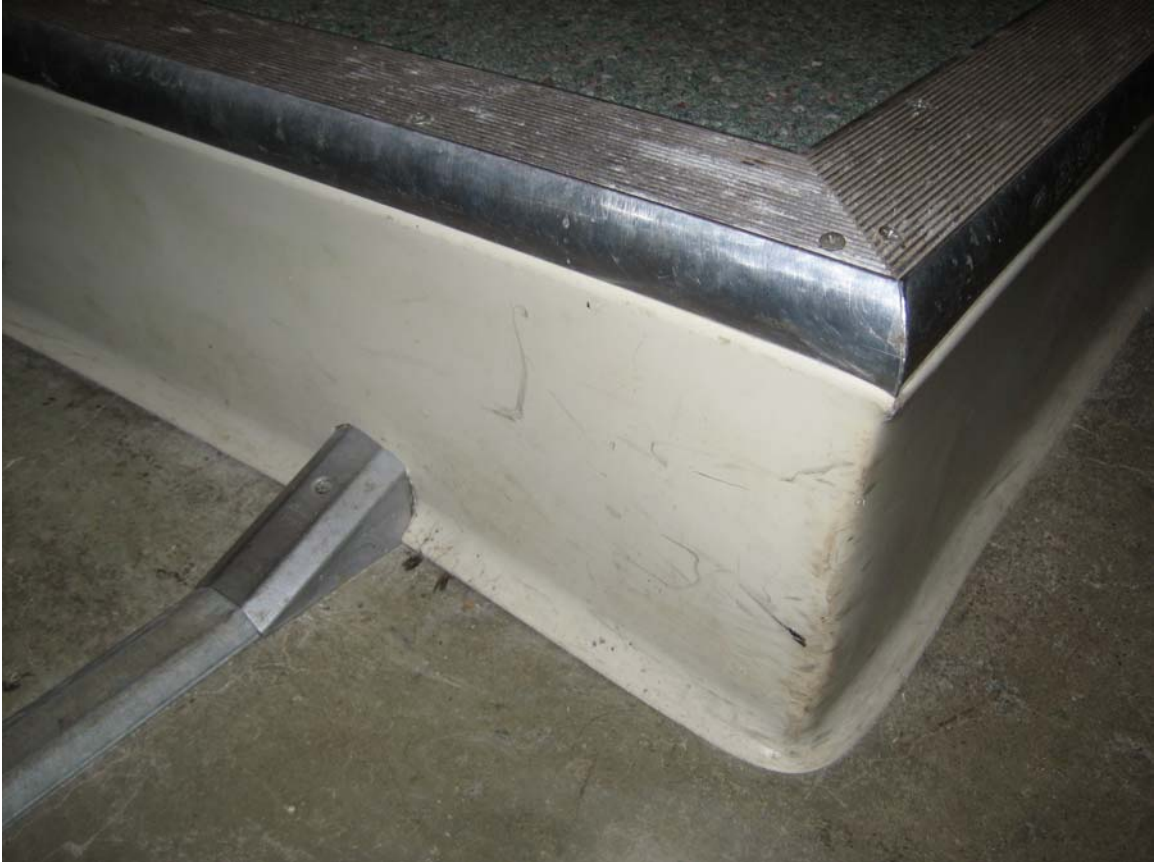
HA #5 – Assumed asbestos containing 6” khaki cove molding and associated mastic
